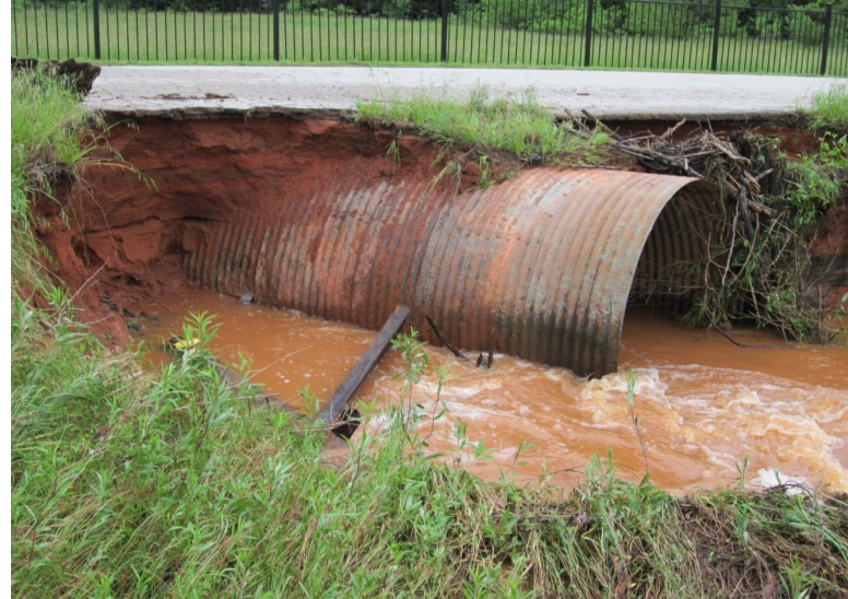
May 2015 Flood – 72 nd Ave NE between Robinson and Alameda
