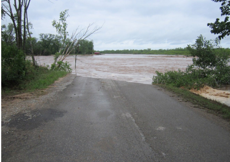
May 2015 Flood – Rock Creek Rd and 72 nd Ave NW
