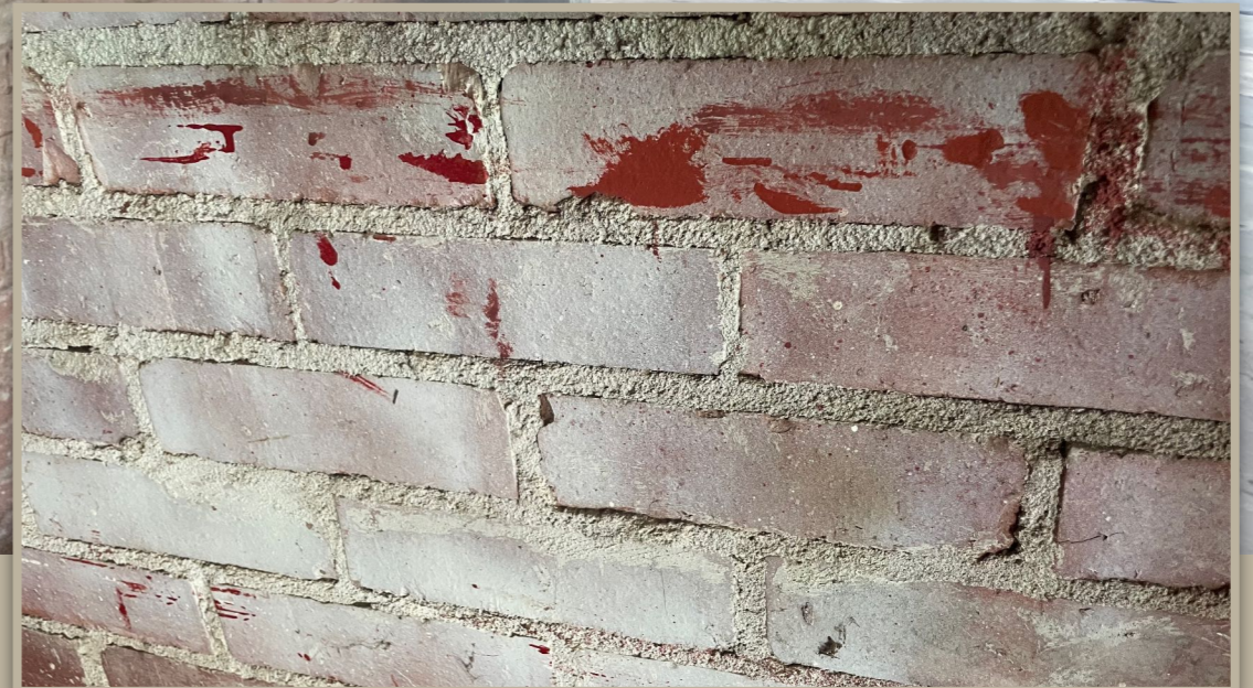
Patched brick & mortar under garage windows?
