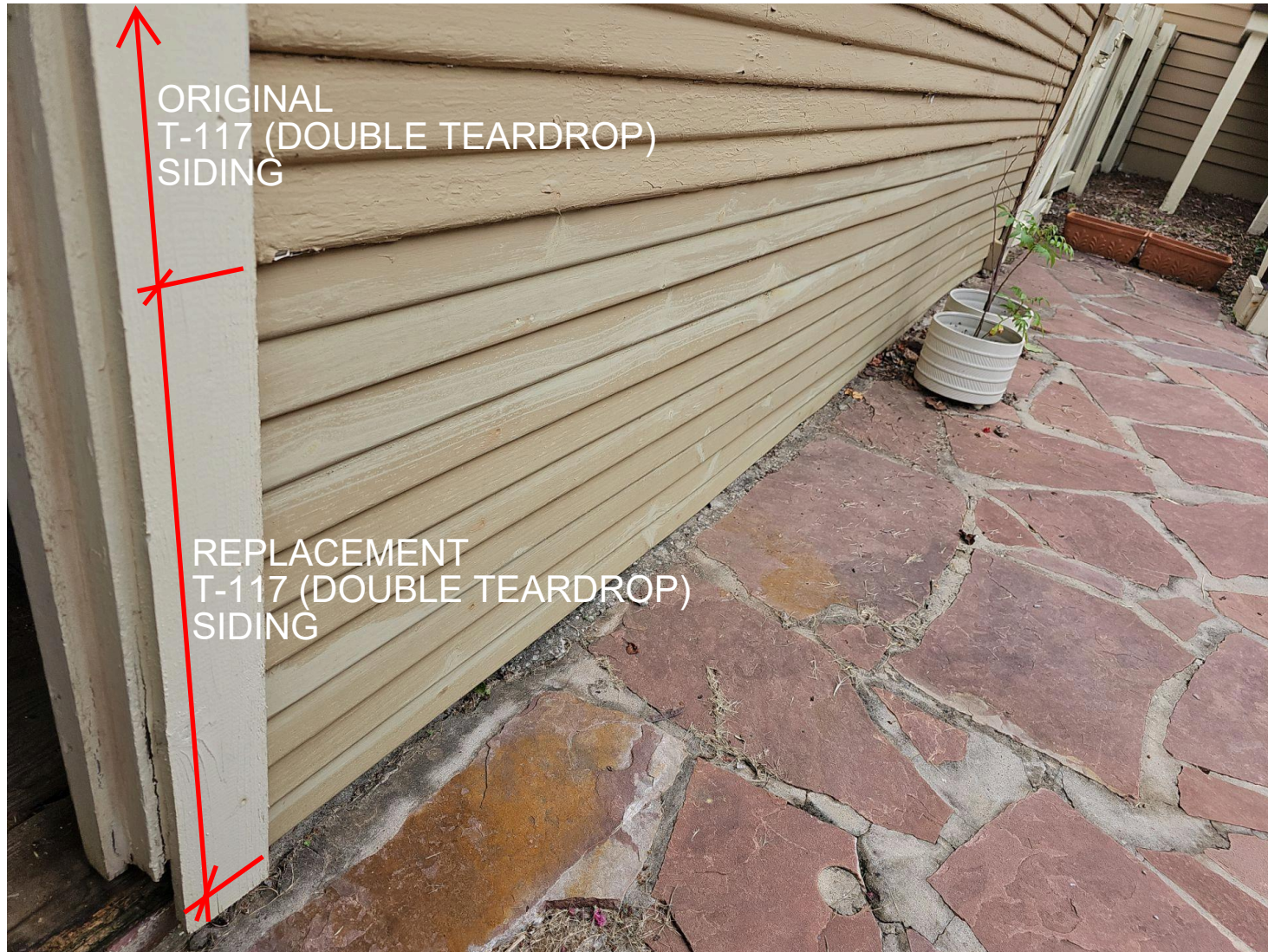
CLOSE UP: AREA OF PREVIOUSLY REPLACED WOOD T-117 (DOUBLE TEARDROP) SIDING
