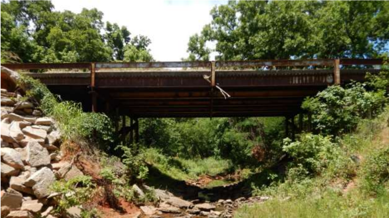
60 th Ave NE Bridge over Rock Creek (located north of Rock Creek Rd).
