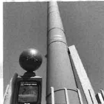
Radiation from 5G tower: .004 W/square meter
