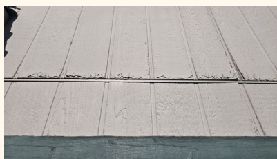
failed paint & water damage
