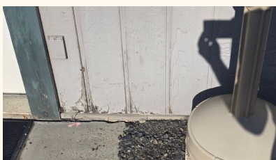
failed paint & water damage
