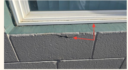
masonry sealant needed
