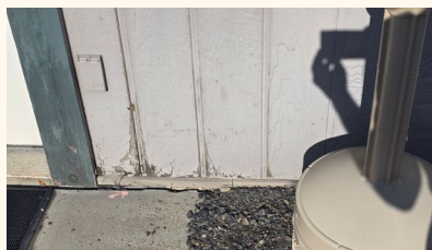
failed paint & water damage
