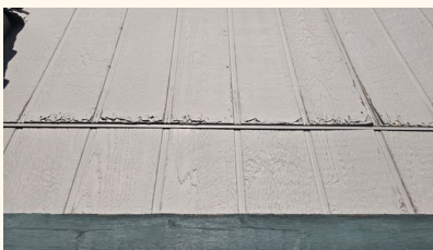
failed paint & water damage
