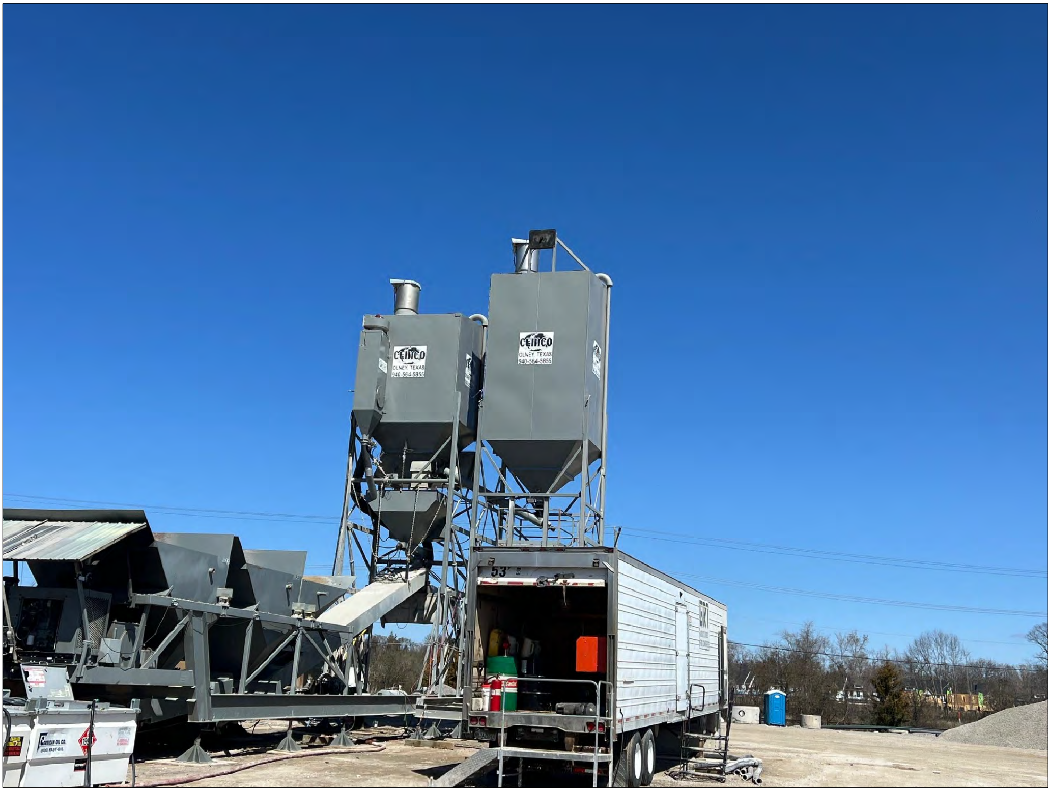
MARK ANTHONY CONCRETE BATCH PLANT SETUP
