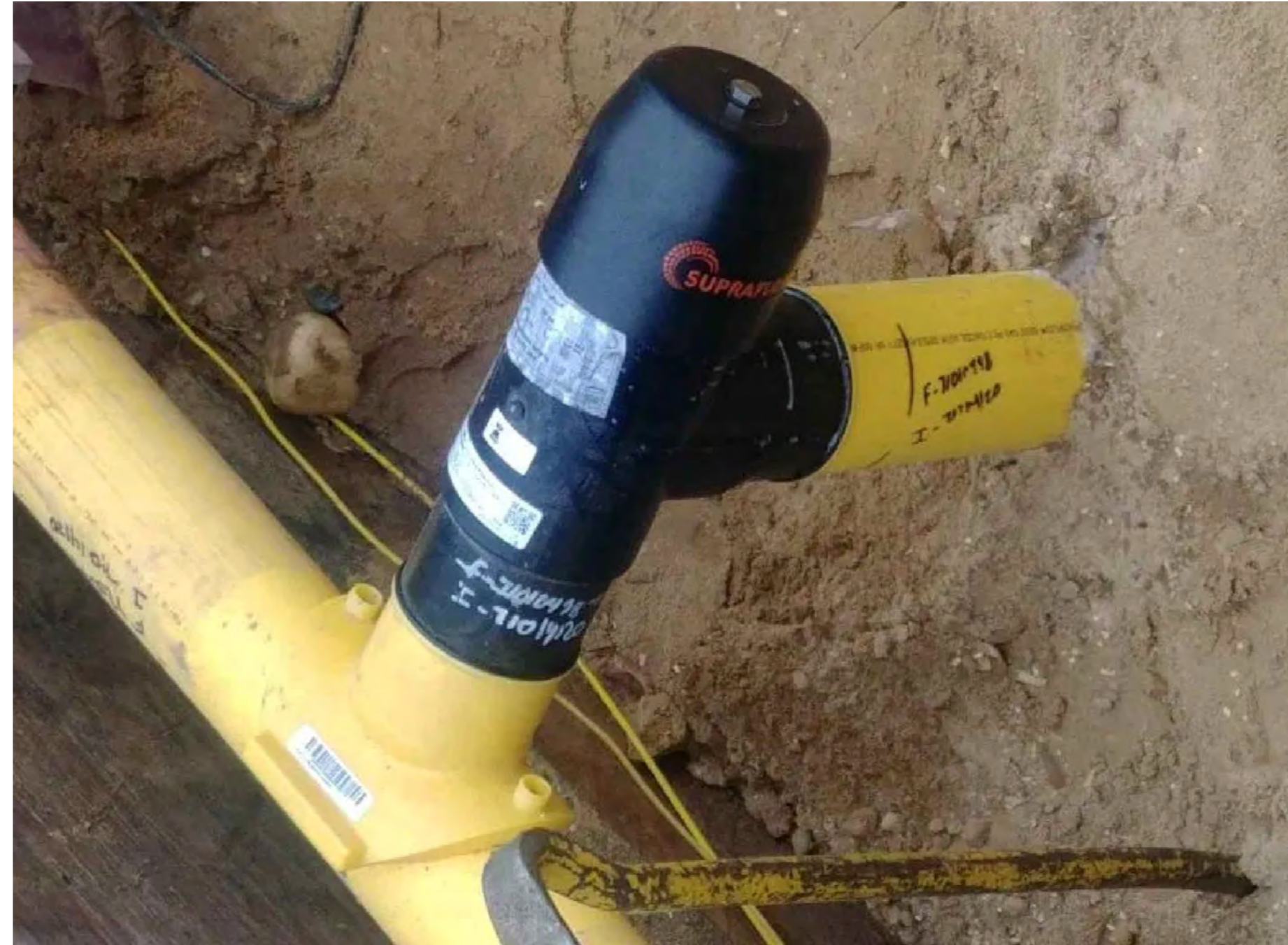
GAS LINE CONNECTION PHOTO
