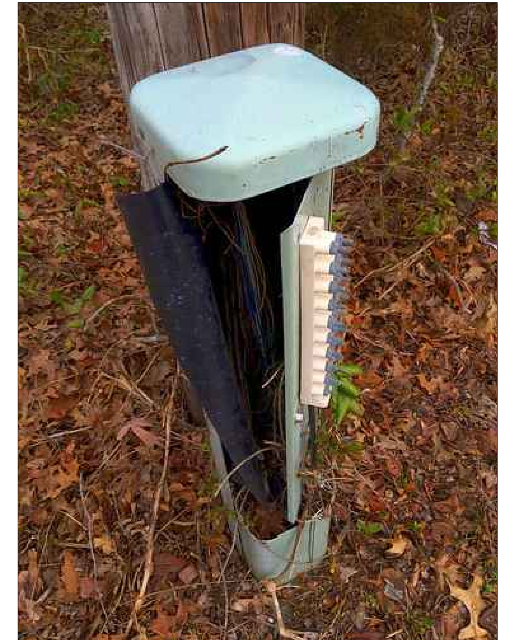
TELEPHONE PEDESTAL CONNECTION PHOTO
