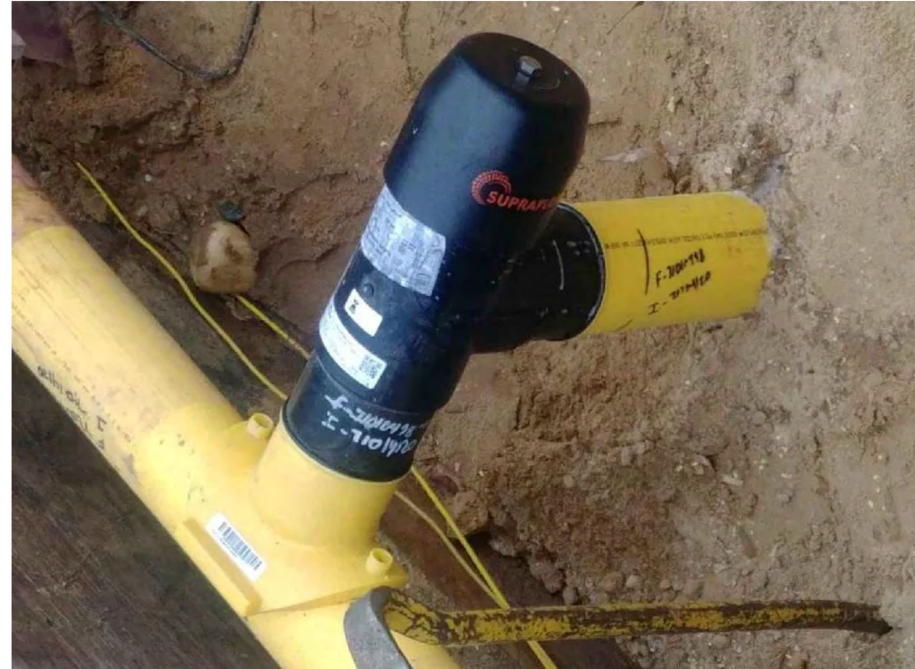
GAS LINE CONNECTION PHOTO
