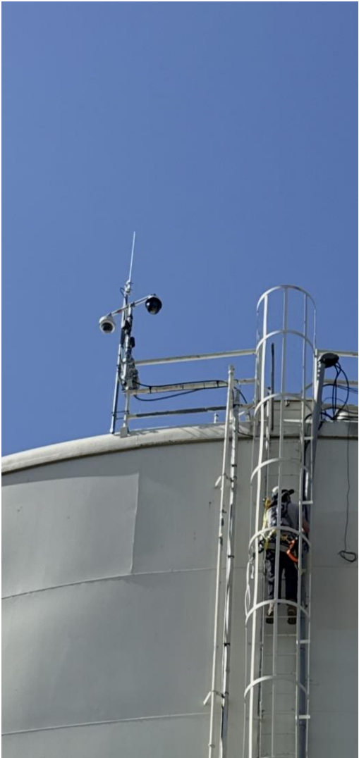
Examples of equipment mounting: Pipe to pipe fittings to existing railings on Upper Tanks
