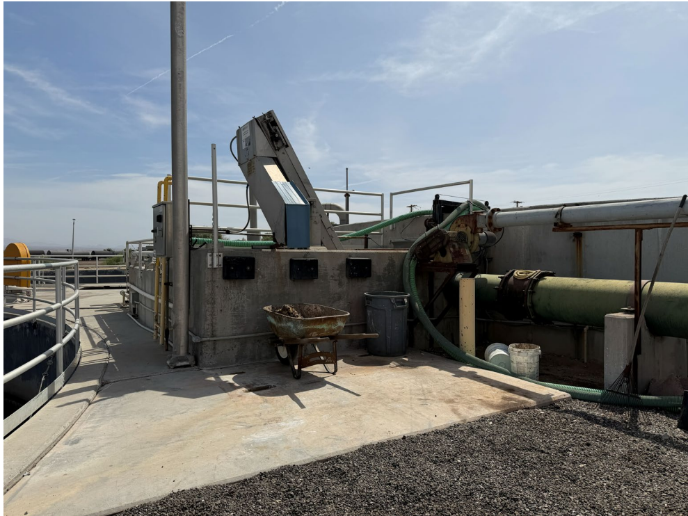
Figure 3. A mechanical bar screen removes larger solids from the influent wastewater. Solids are collected in the wheelbarrow and hauled.
