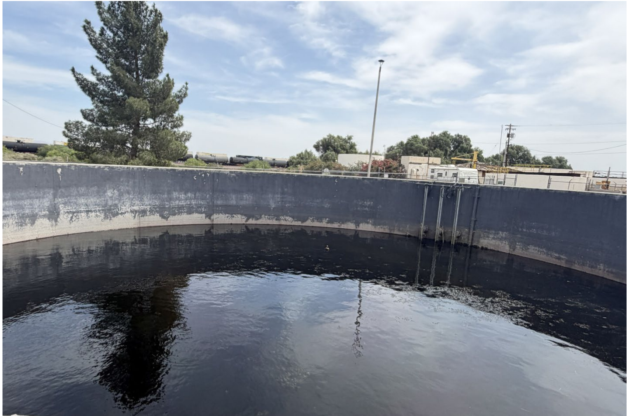
Figure 9. The effluent equalization basin stores treated wastewater. Treated wastewater from the effluent equalization basin is pumped to the evaporation/percolation ponds.
