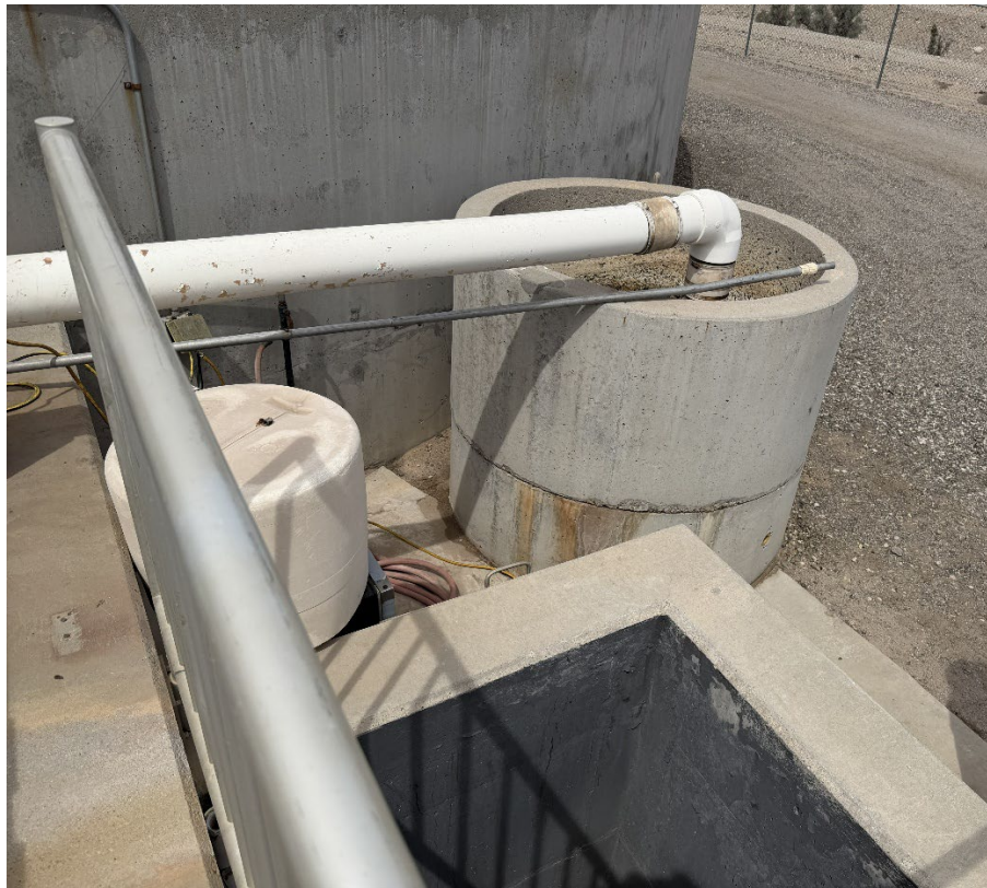
Figure 8. The effluent wet well shown in the foreground. Effluent samples are taken from the effluent wet well using an automated composite sampler located to the left. In the background a wood chip basin is used for odor control.
