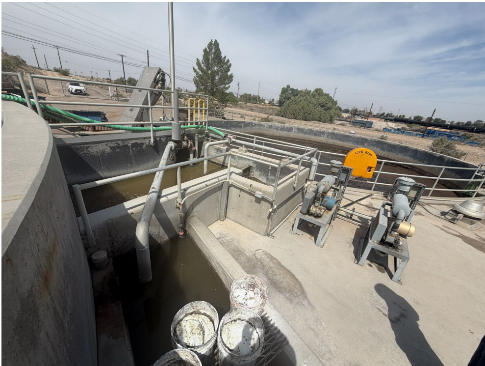
Figure 4 The aerated grit chamber that utilizes an airlift pump that operates 24 hours a day. Grit is collected in 5-gallon buckets, and lime is placed on top to help limit vectors and odors.
