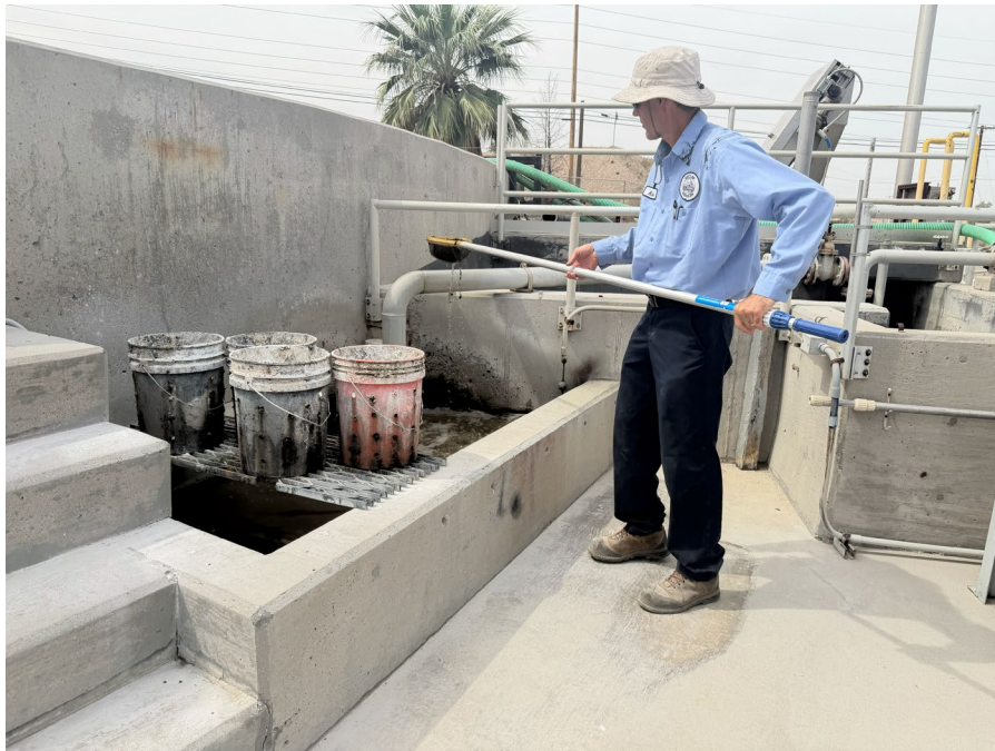
Figure 5. The airlift pump is in operation, and the operator is scooping out grit from the grit settling zone and placing the collected grit in the five-gallon buckets.
