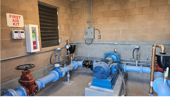
Booster Pumps and Plumbing
