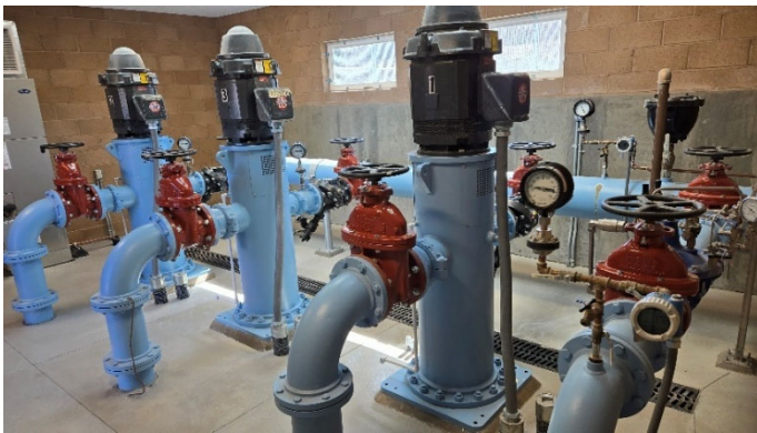
Booster Pumps and Plumbing
