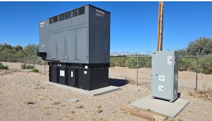
Phase 4A: Emergency Generator at Well 11
