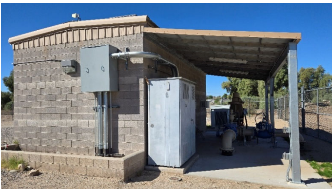
Treatment Building with Shade Structure for Well 15
