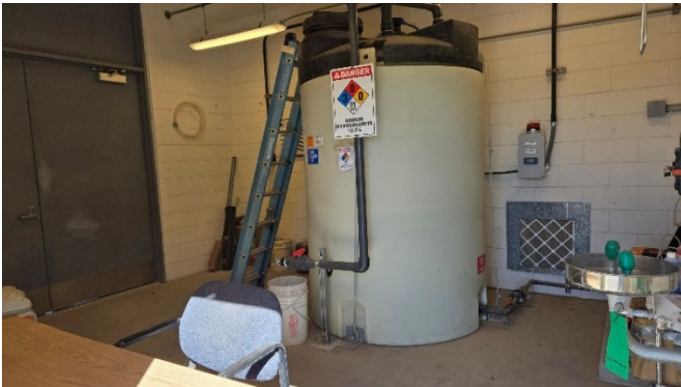
Sodium Hypochlorite Tank
