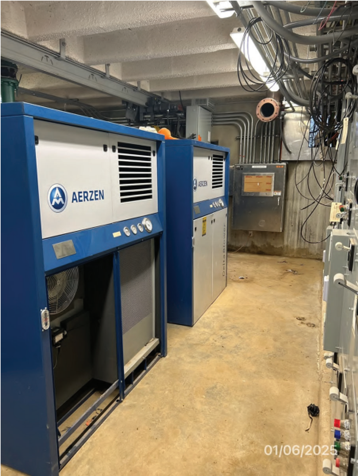
11. Process blowers and electrical gear
