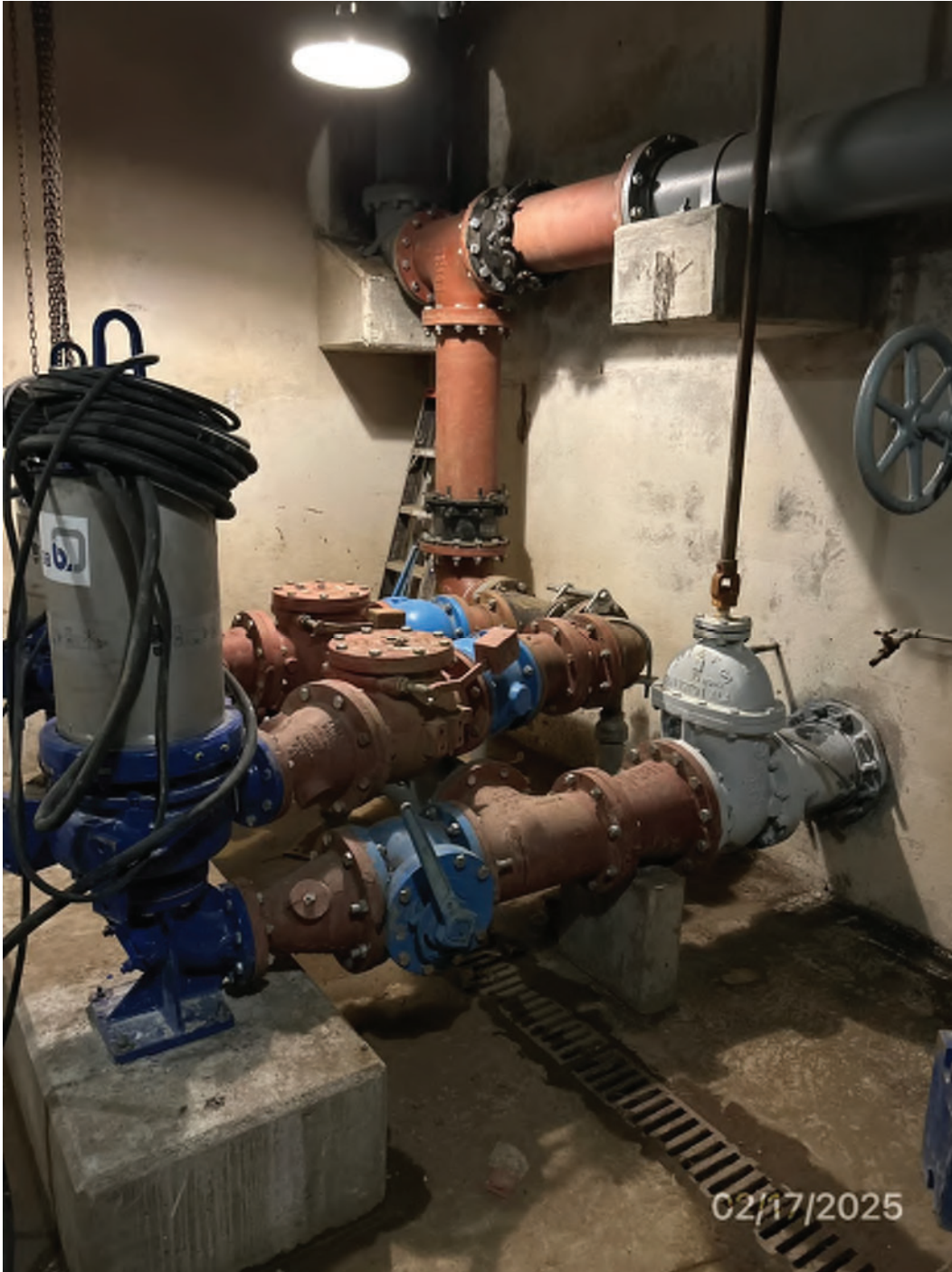
1. New influent pumps and piping
