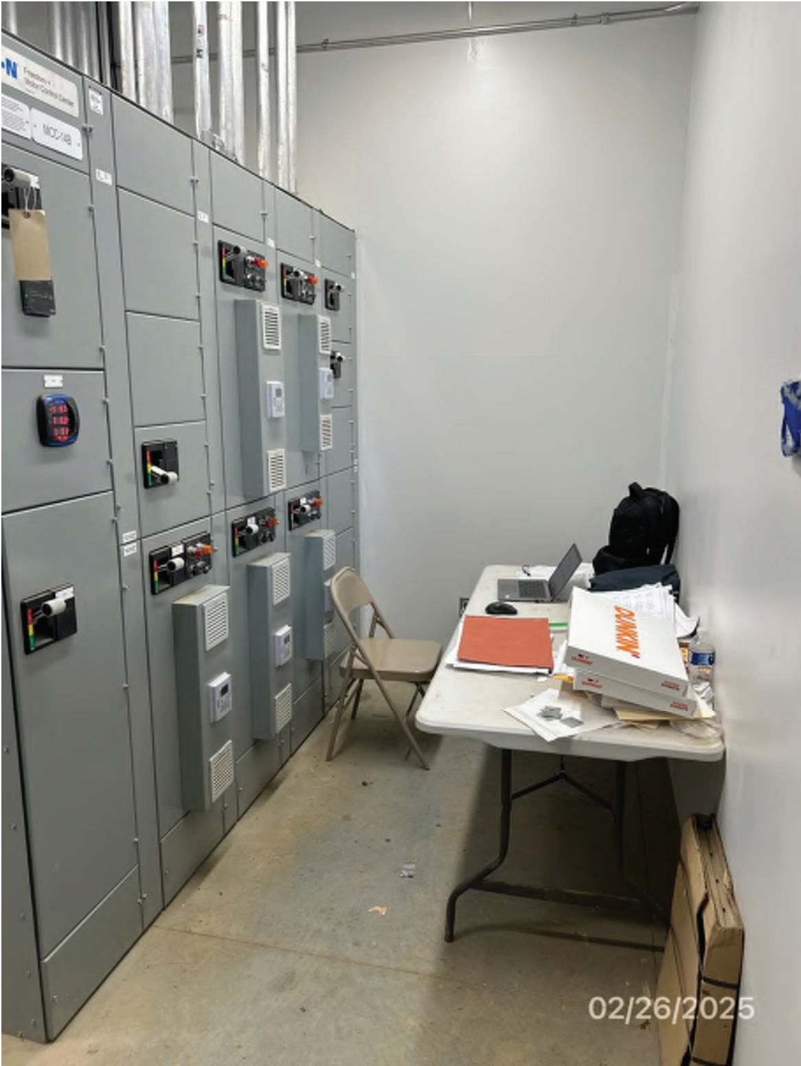
10. Membrane electrical gear
