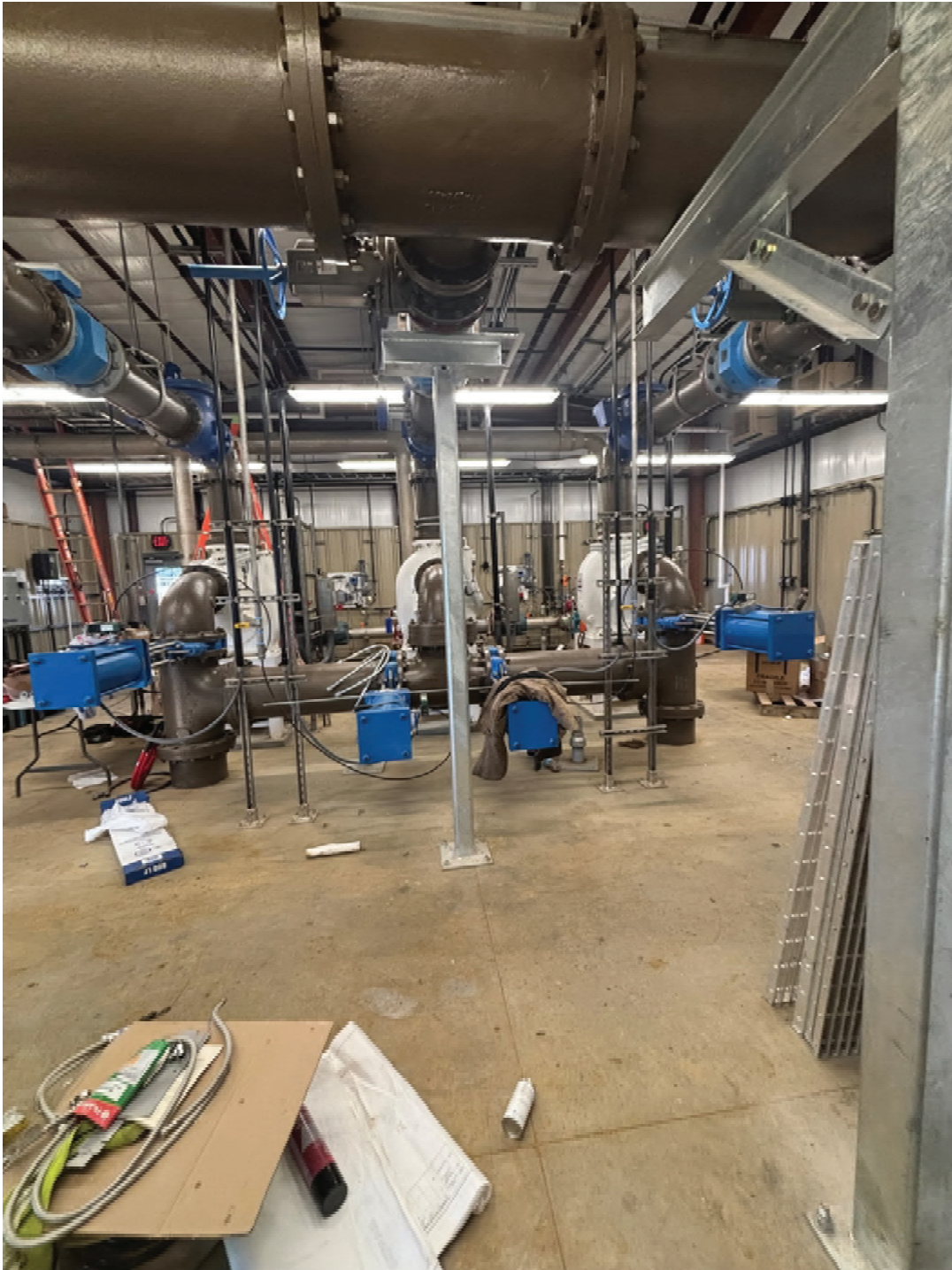
7. RAS pumps and piping
