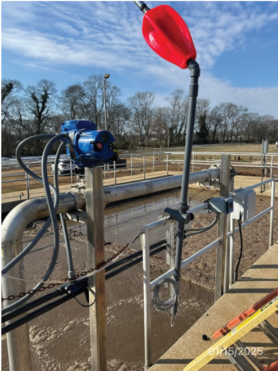
3. Treatment basin 1 with baffle wall, new air piping and control valve, and instrumentation.
