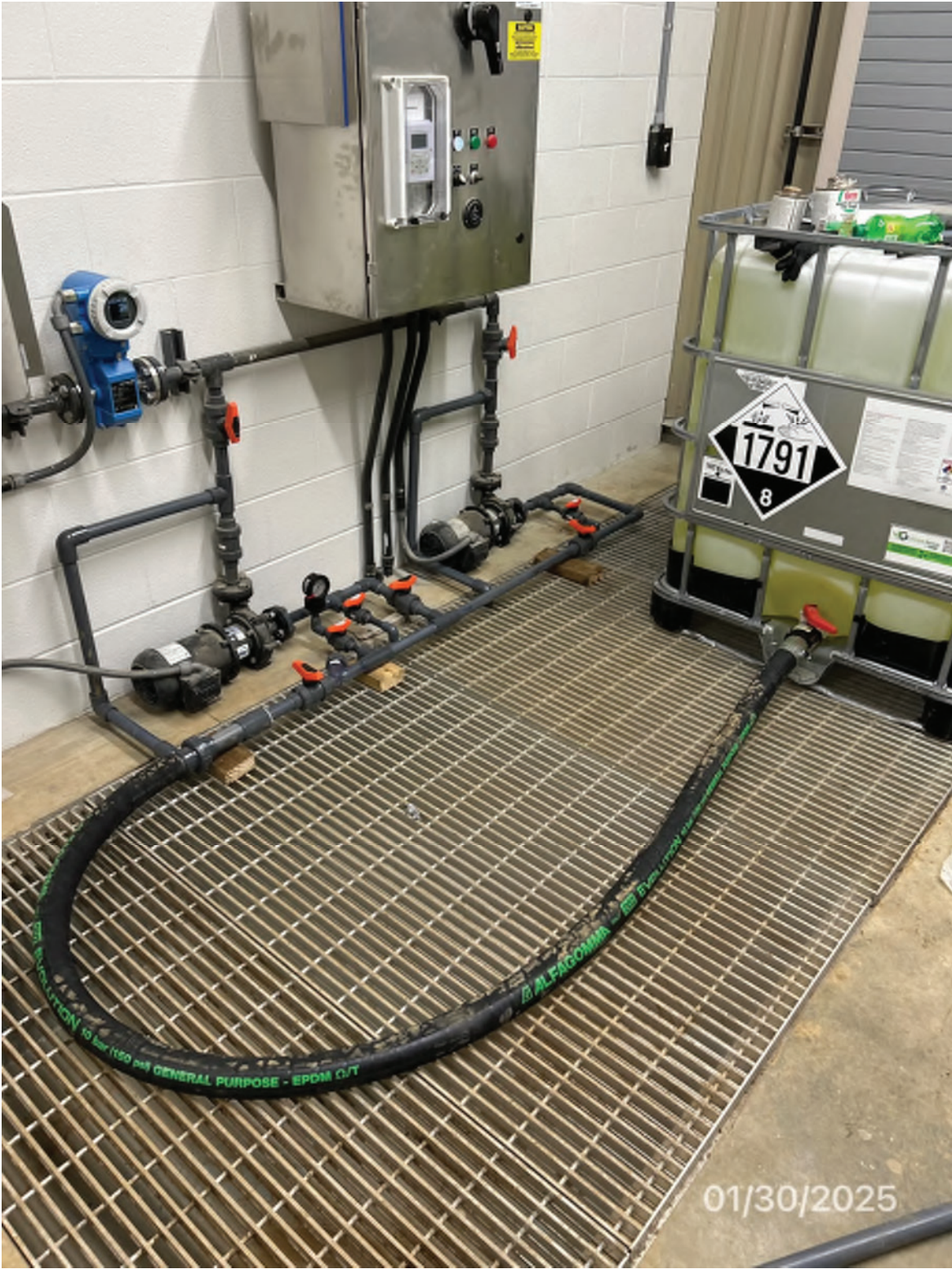
9. Membrane chemical feed
