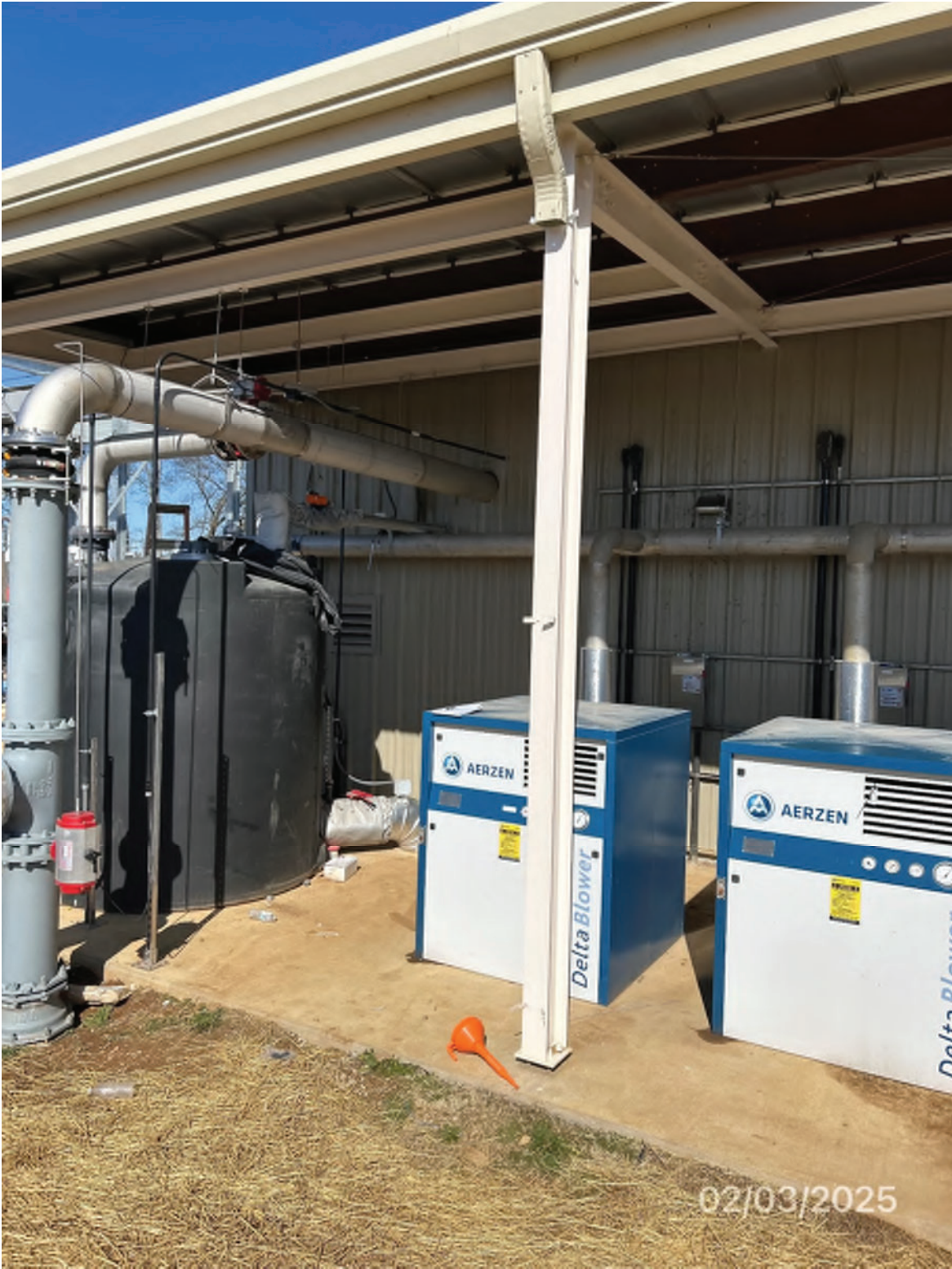
8. Membrane backpulse tank and blowers
