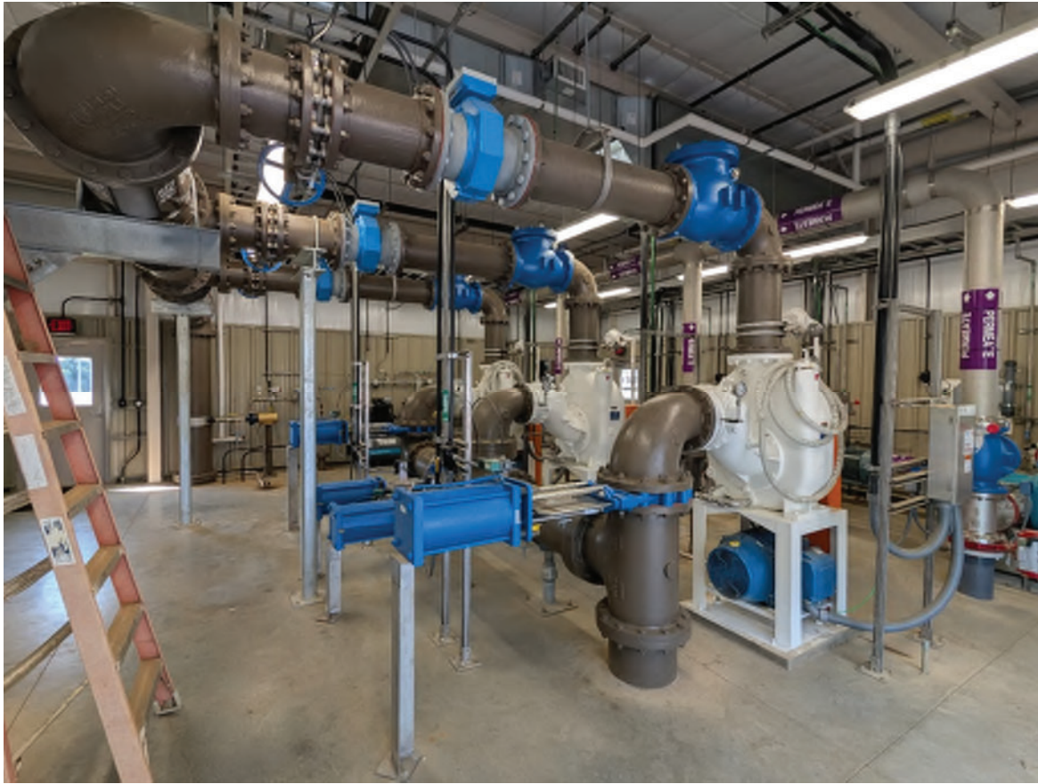
9. MBR RAS pumps
