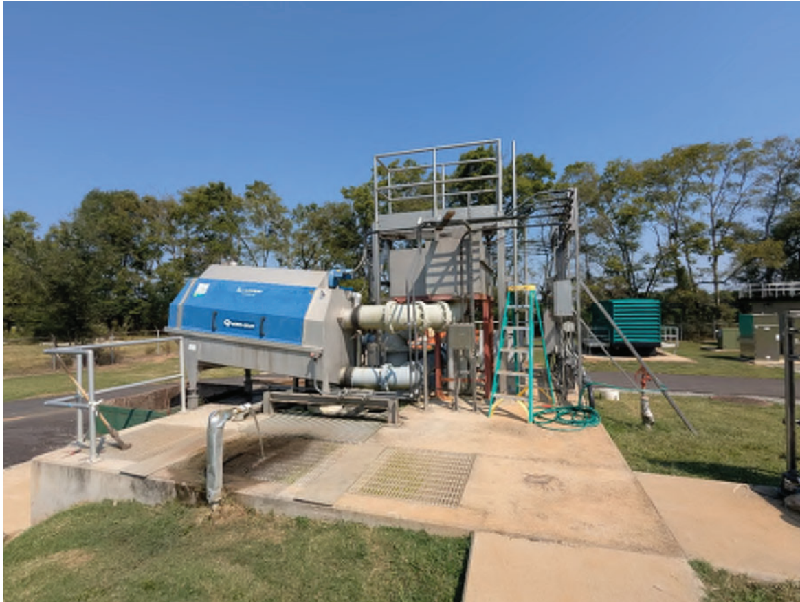
3. Headworks with fine drum screens
