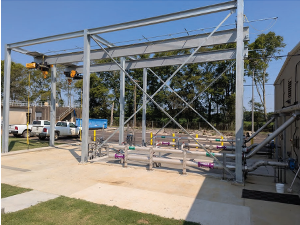
1. MBR basins with overhead hoists
