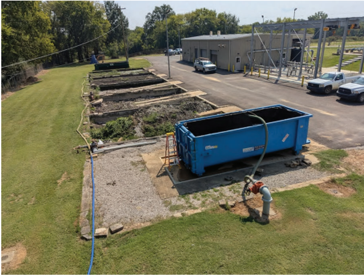
6. Sludge dewatering box and drying beds
