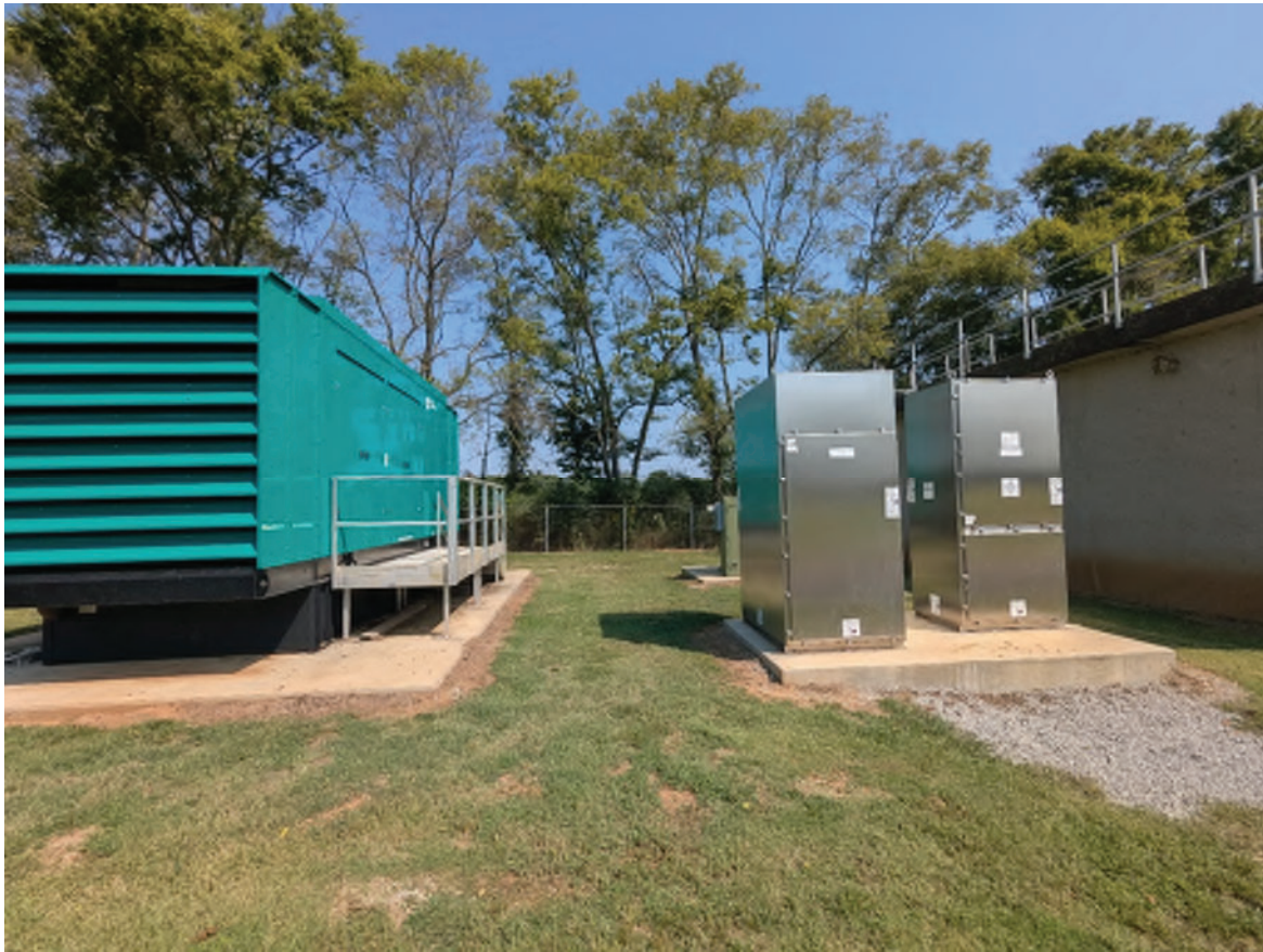
4. Generator and Automatic Transfer Switches
