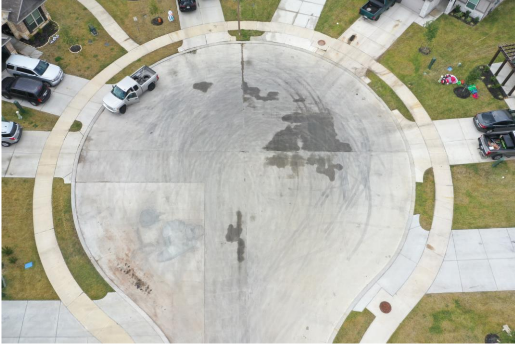
48 hours post-flooding (Before Repair)
