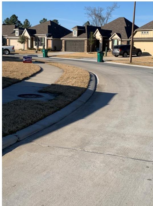
48 hours post-flood (Post Repair)
