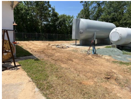
Figure 2: Hydropneumatic Tanks May 17, 2022
