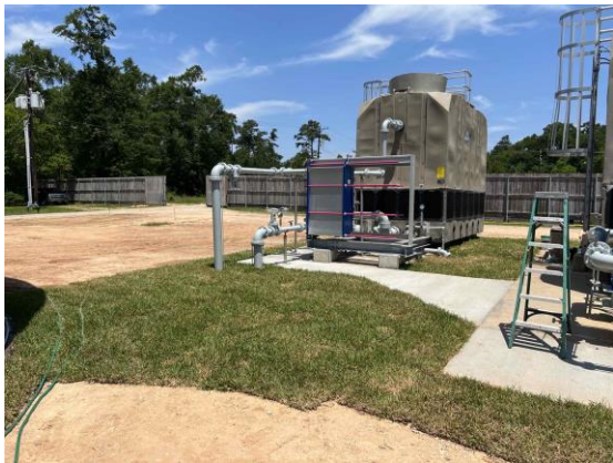
Figure 1: Cooling Tower May 17, 2022
