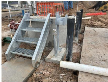
Well Head of the Lift Station February 9 th
