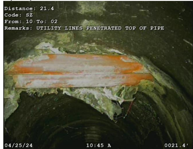
Figure 3: Utility Line Penetration
