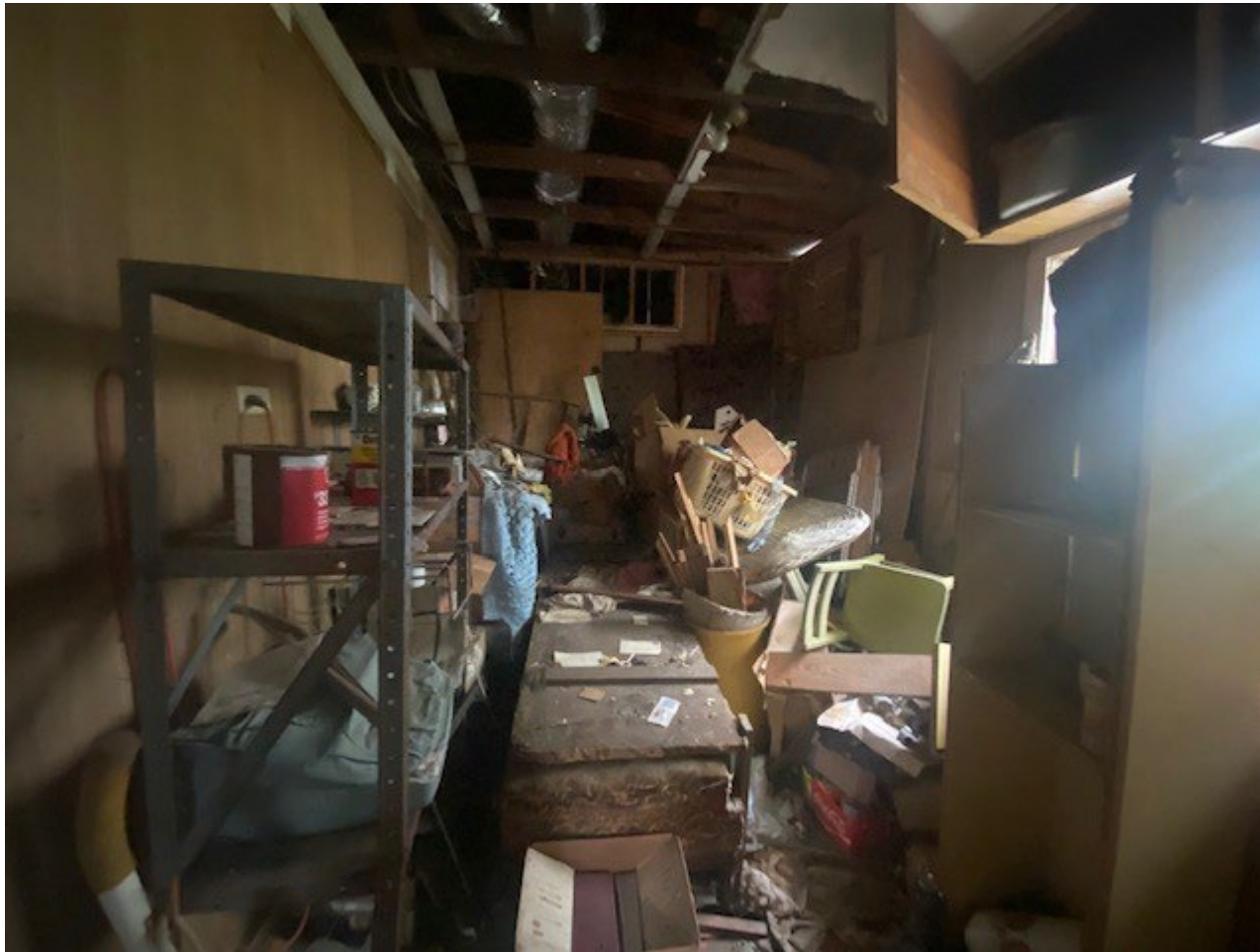
The 2 nd addition to the original home. The ceiling has fallen due to water intrusion, massive frame and subfloor damage.
