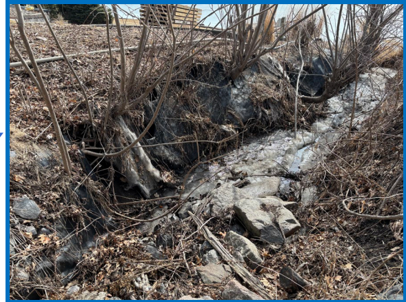
Figure 4. Erosion in the channel in the fire lane (looking south)
