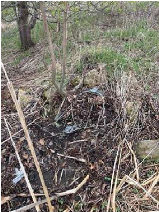
Figure 14: 15" RCP Inlet (S)
