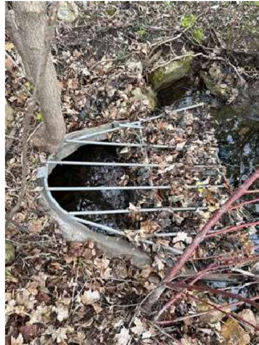
Figure 9: 24" RCP Inlet (S)
