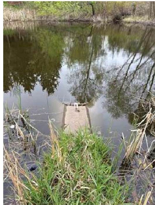
Figure 6: 21" RCP Inlet (E)
