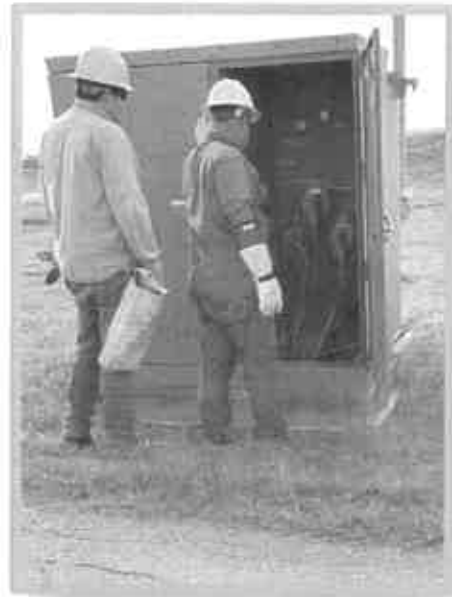
AEP Checking Electrical Surges
