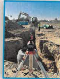
4 th Street / Dunlap Collapsed Manhole Replaced 15" Sewer Line Replaced
