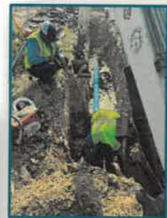
Lee Street Sewer Tap
