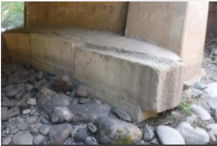
A Observed scour at Pier 2 exposed footing
