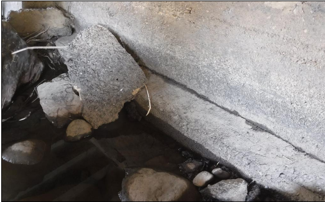
Abutment 5 exposed footing near mid length.
