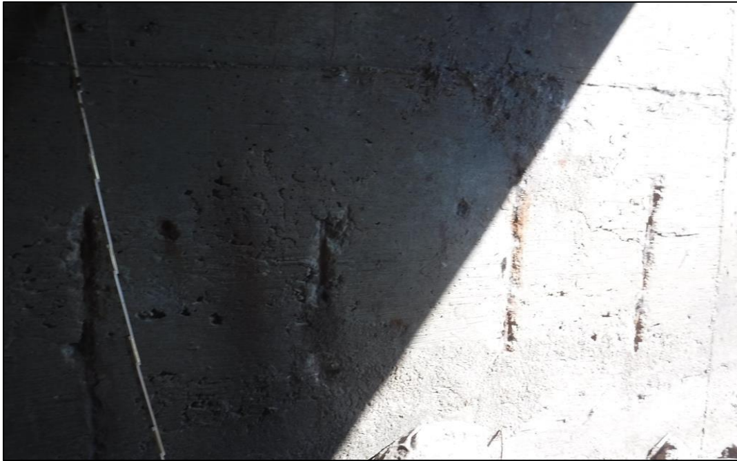
Abutment 5 has 5 locations of exposed rebar.
