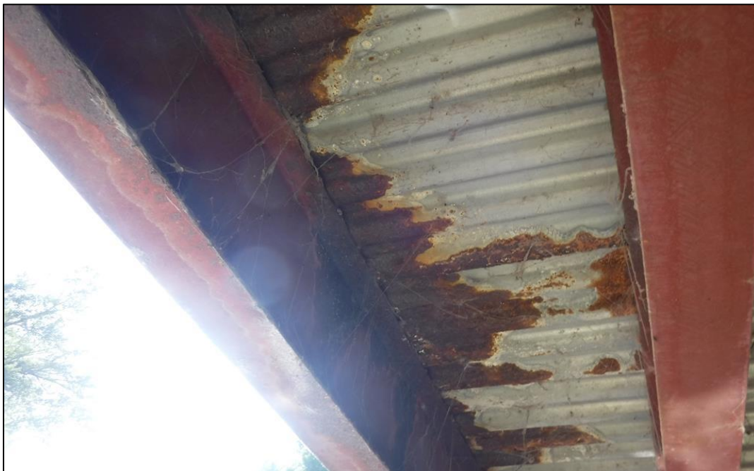
Girder 4K has heavy corrosion.
