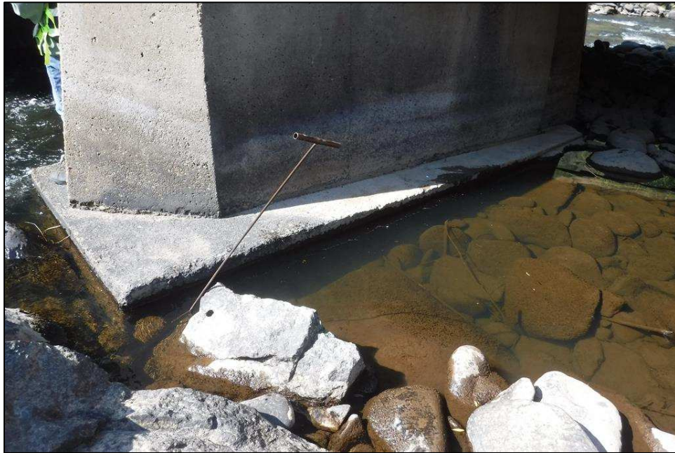
P4 north side exposed footing.
