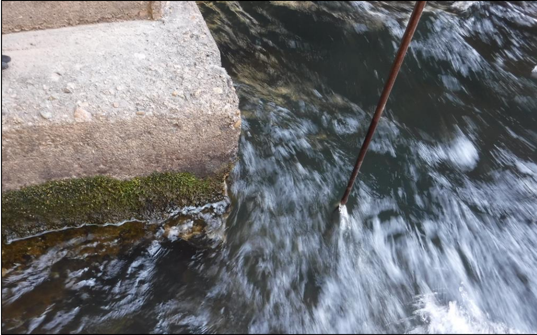
P4 scour hole at SW corner upstream side.
