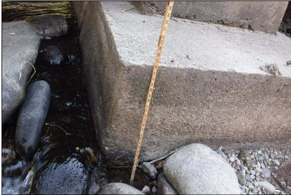
P3 exposed footing at downstream end.
