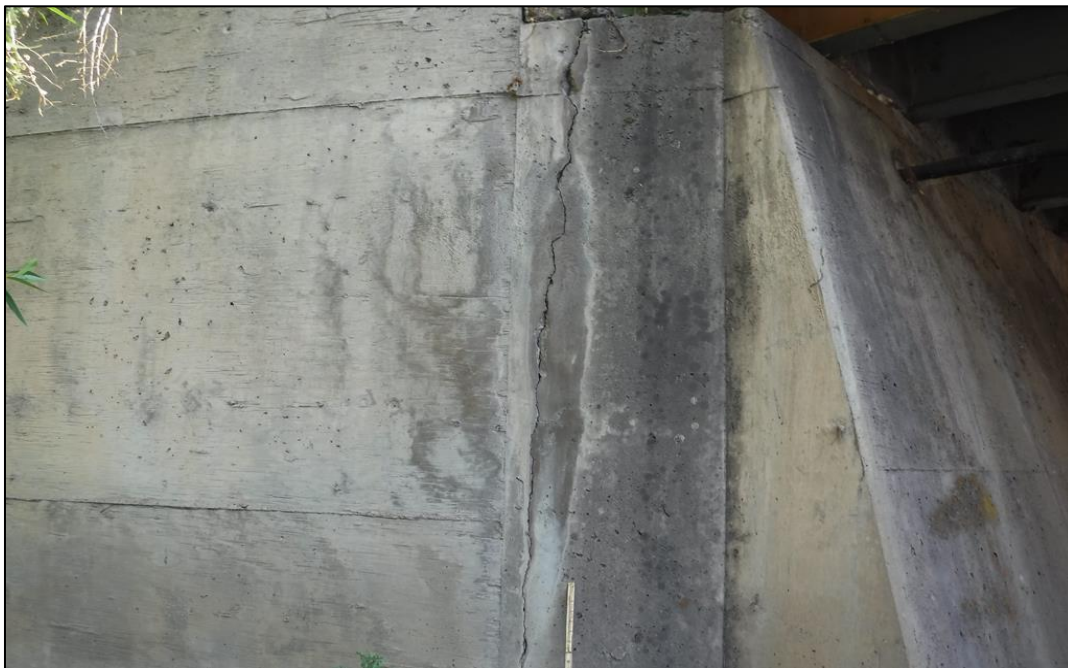
NW wingwall has a vertical crack at Abutment 5 joint.
