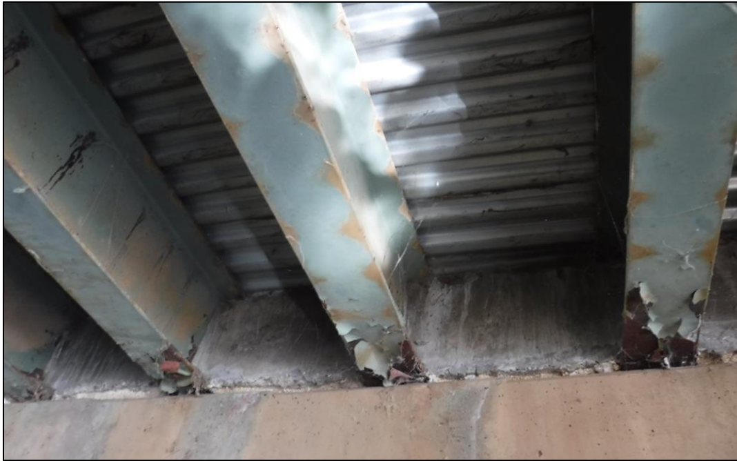
Peeling paint with corrossions at ends of Girders A to K at Span 5.
