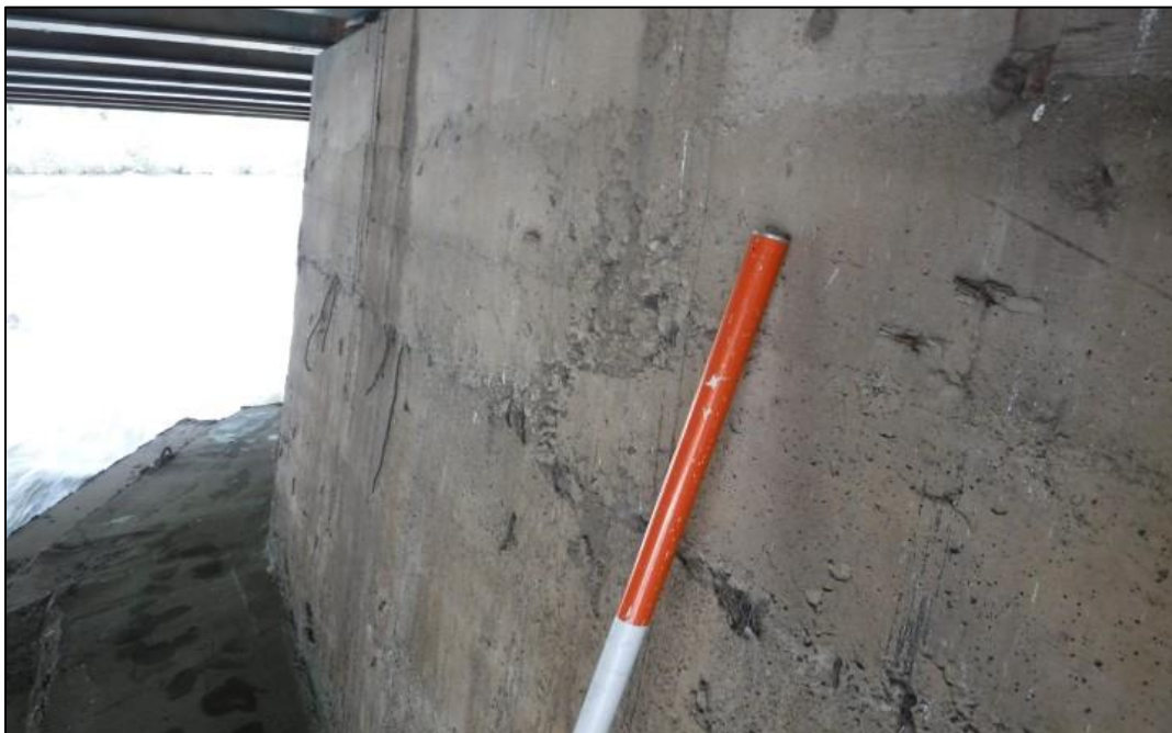
Honeycombs at Pier 2.
