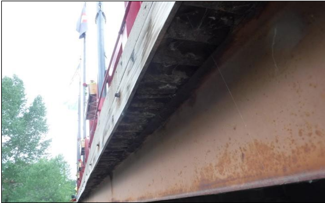
Failed deck forms and desintegrating deck along east overhang in Span 4.
