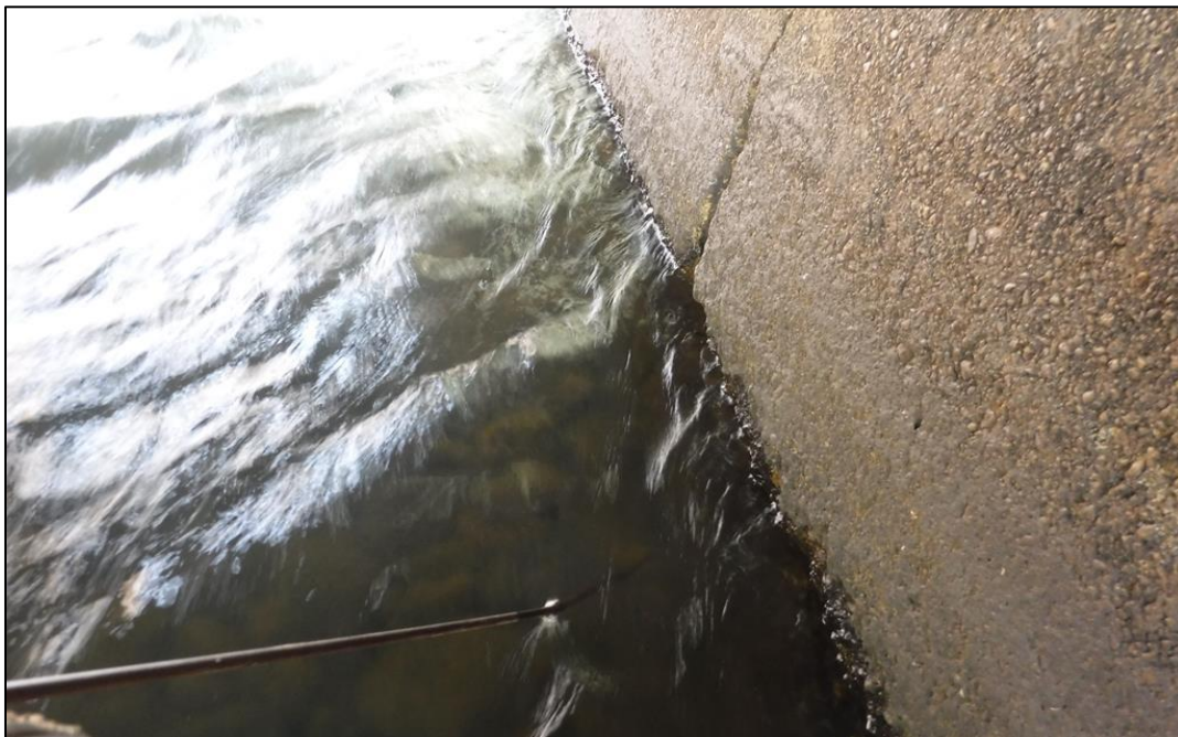
P3 undermined footing at upstream south side.
