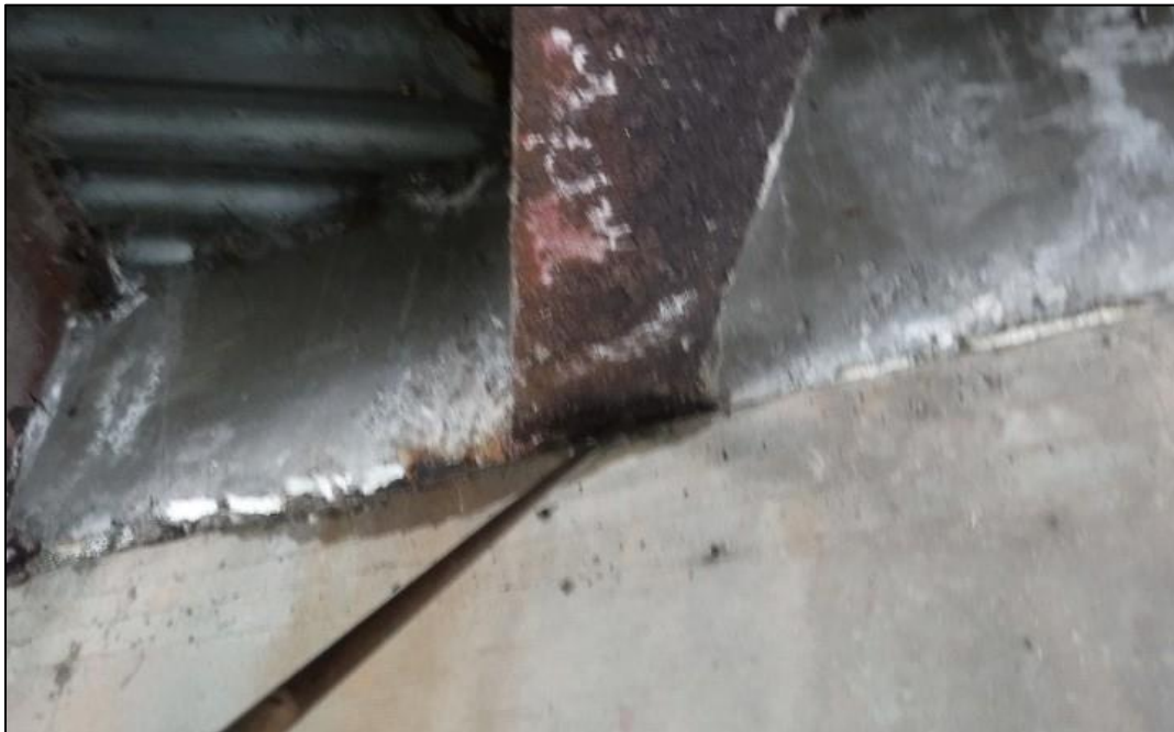
Flaking rust and section loss in bottom flanges of Girders L, M, and N.
