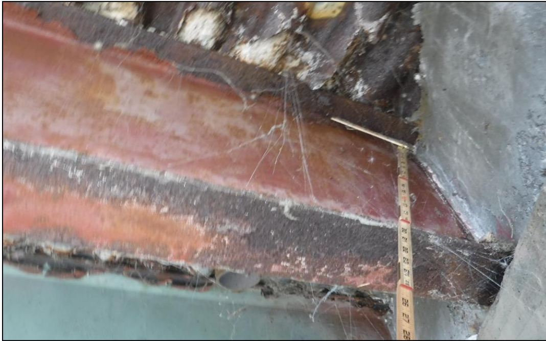
Girder 4L has heavy corrosion.
