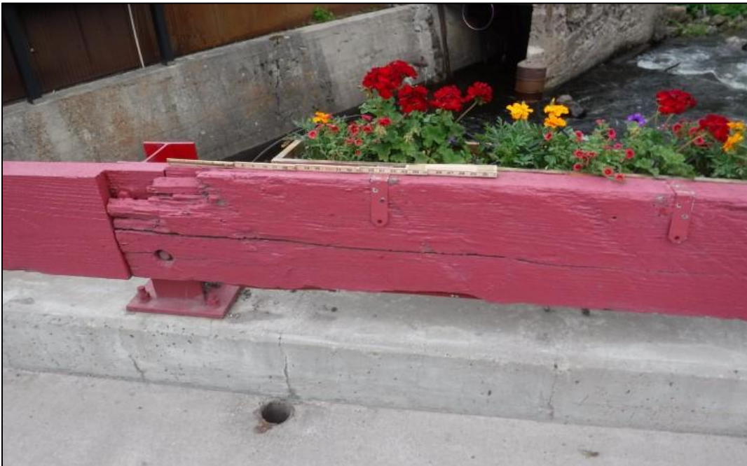
West timber rail broken plank.
