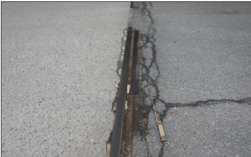
General view of damaged joint armor at N joint-Typical debris in joint.
