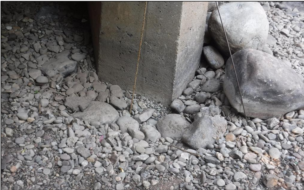
Pier 2 scour at downstream side (2 of 2).
