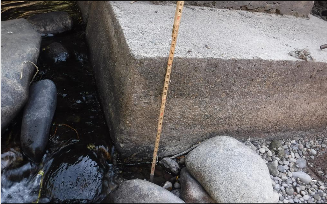
P3 exposed footing at downstream side.
