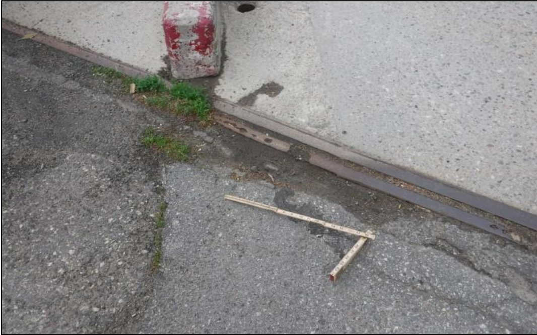
Broken and settled asphalt in walkway at NE corner of deck.
