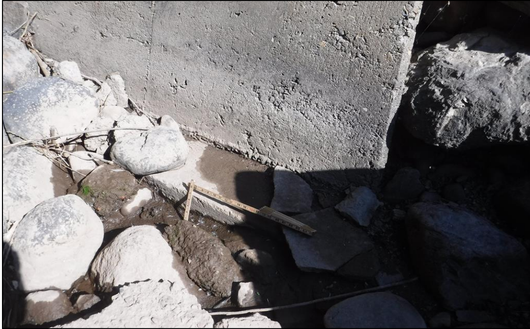
Abutment 5 exposed footing at downstream side.
