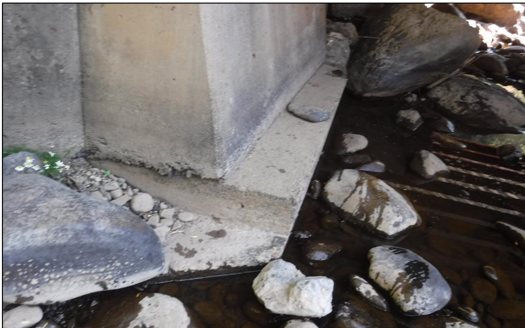
Abutment 5 exposed footing at northwest corner.
