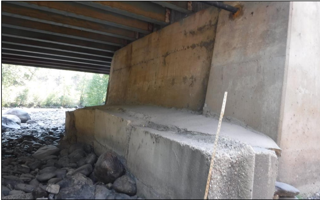
Scour around Pier 2 footer (1 of 2).
