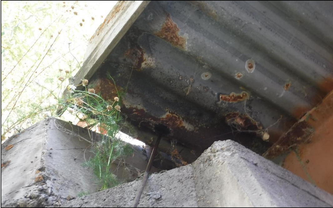
Metal deck has a hole at the northwest corner.
