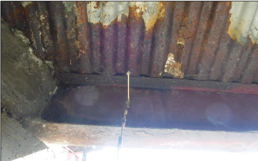
Metal deck at Bay 4N has corrosion.
