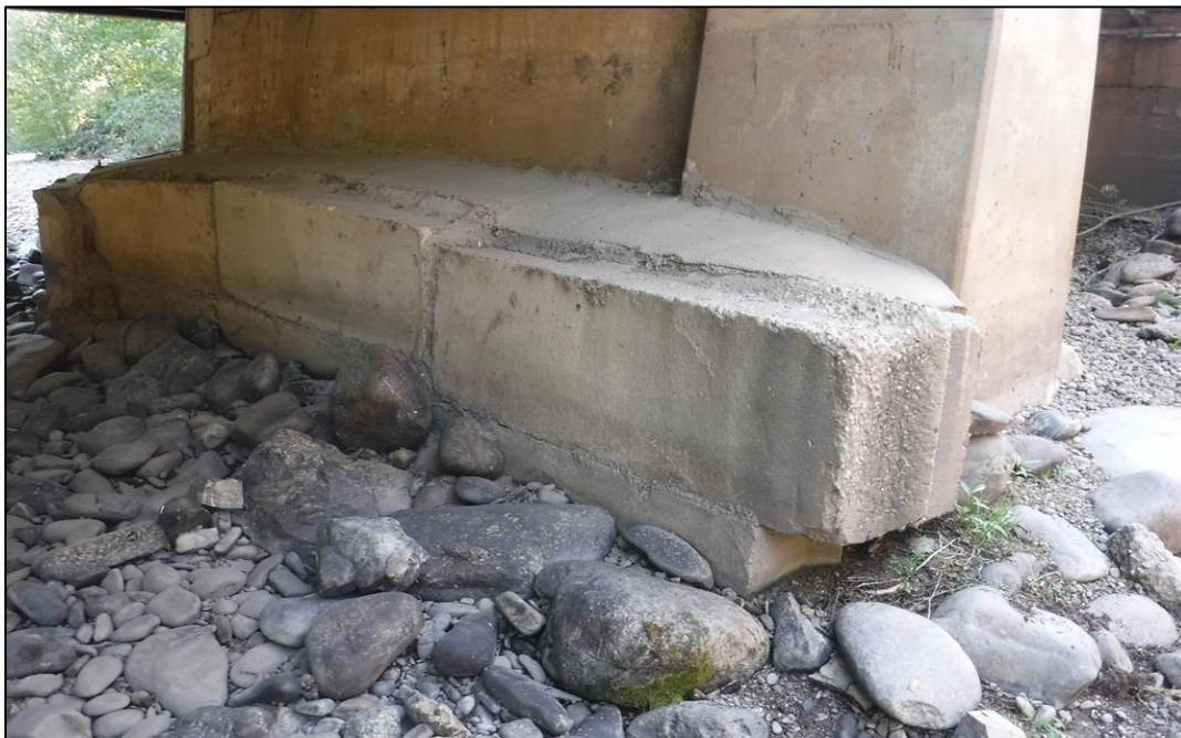
Scour around Pier 2 footer (2 of 2).
