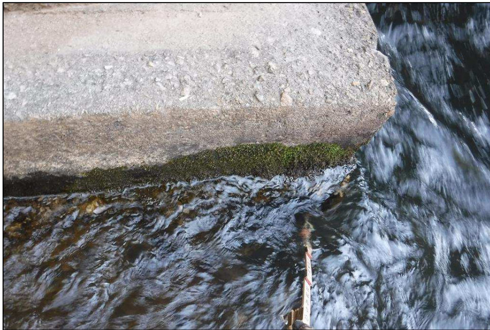
P4 southwest corner undermining at upstream end.
