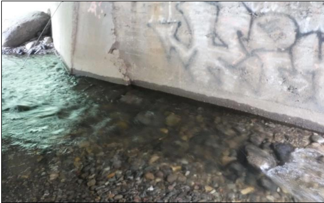
General view of scour in front of A1.
