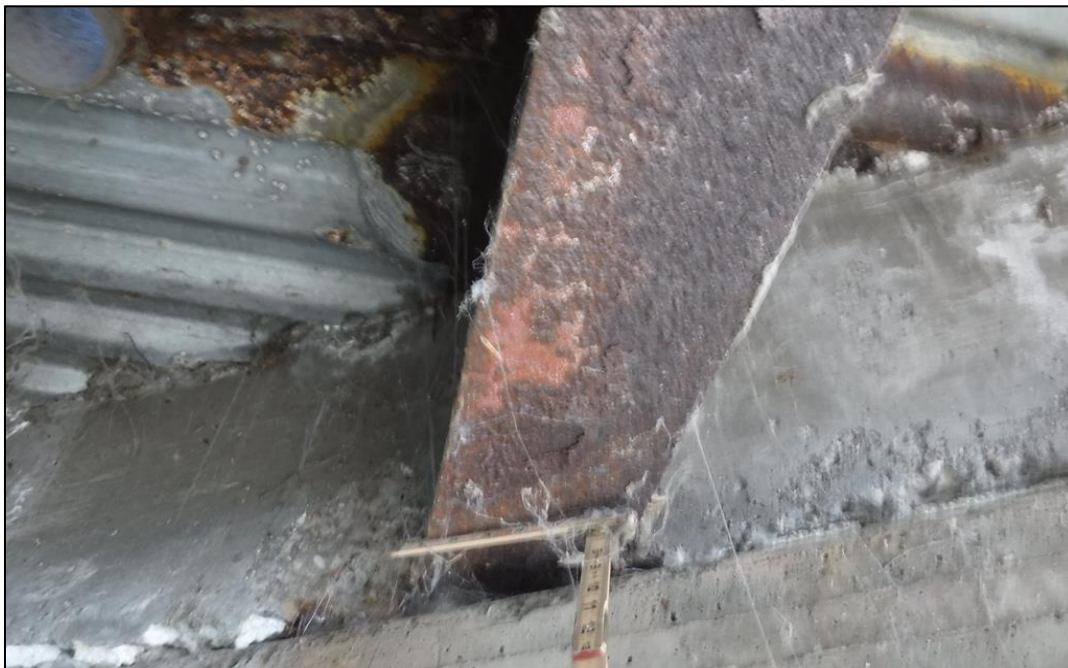
Girder 4M has heavy corrosion.
