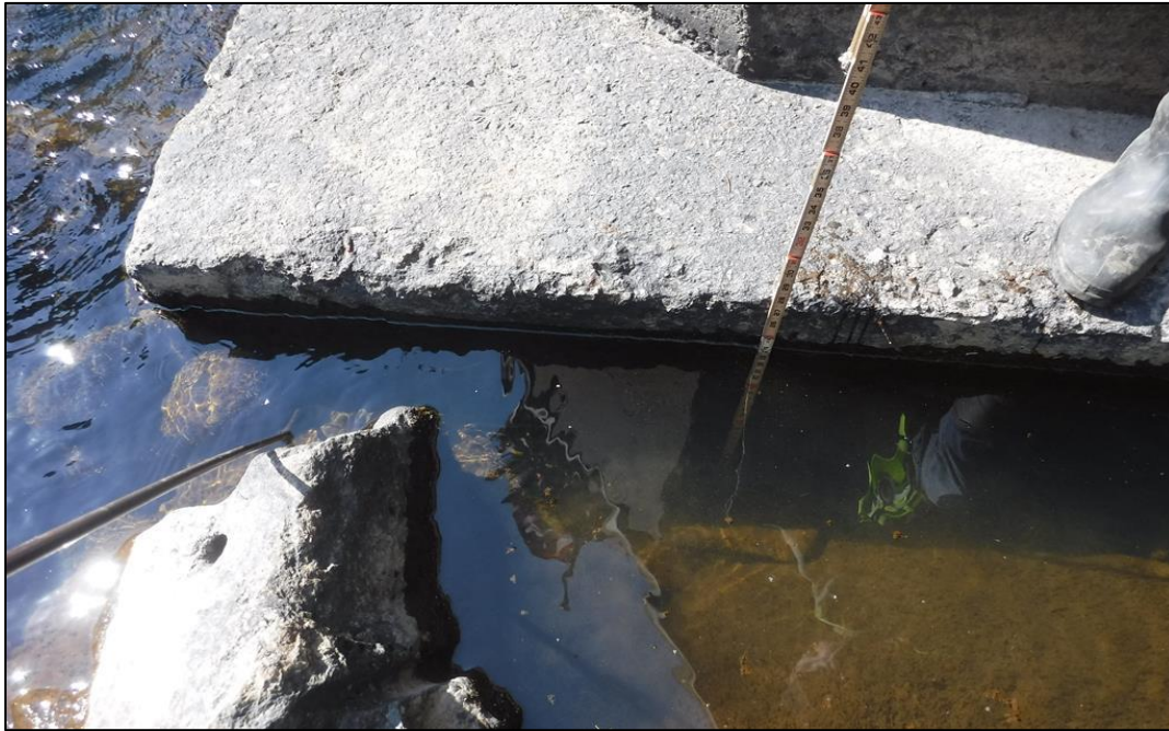
P4 exposed footing at northwest corner.
