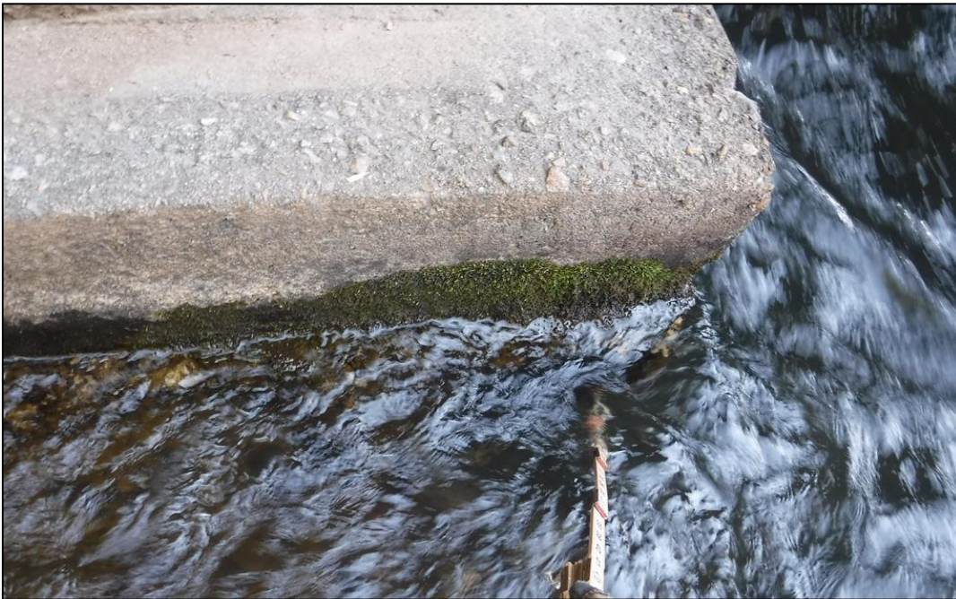
P4 undermining at SW corner upstream side.
