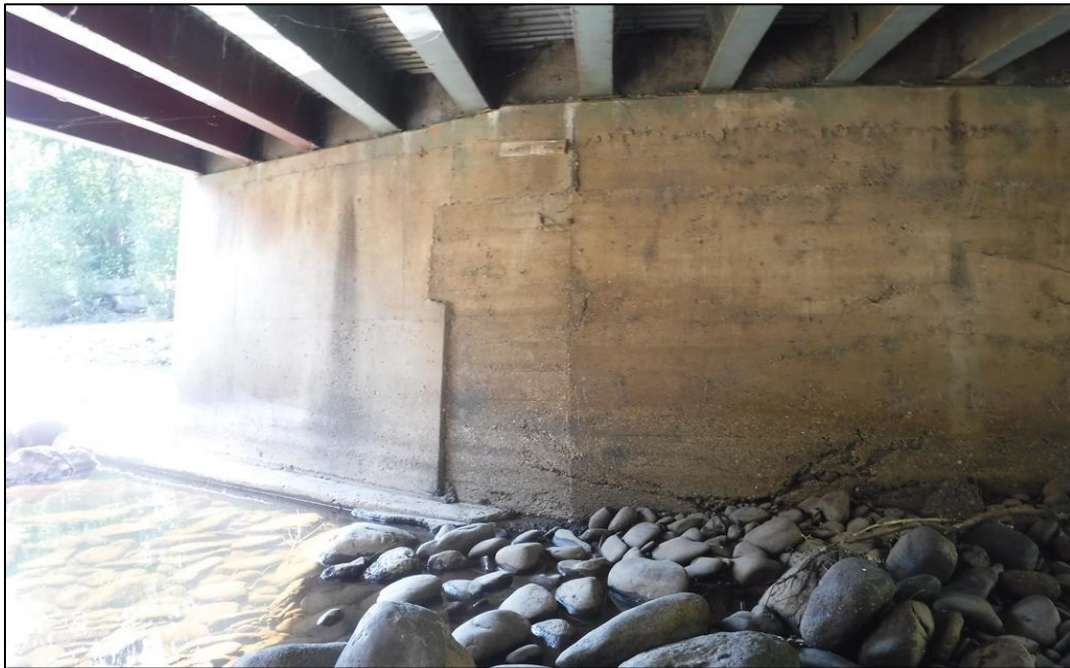
Abutment 5 exposed footing at mid section.
