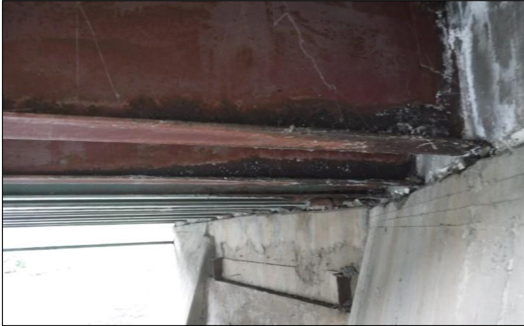
View of corrosion at ends of Girder 4K.
