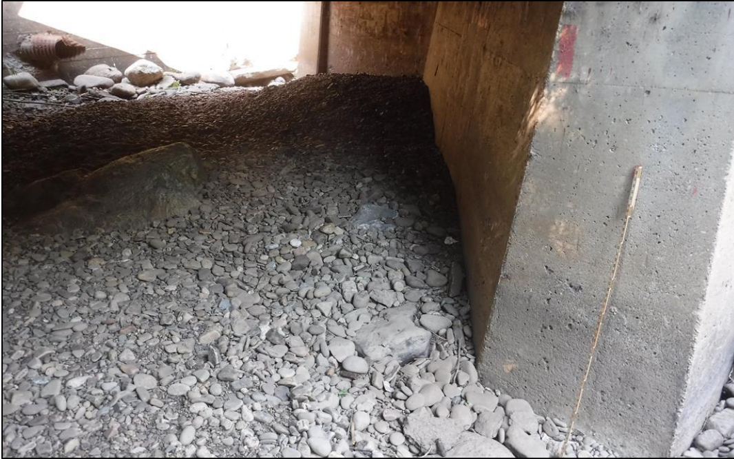
Pier 2 scour at downstream side (1 of 2).
