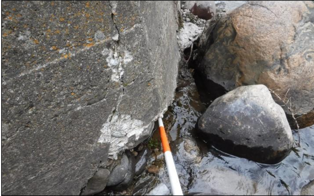
Close up view of undermining at SW retaining wall.
