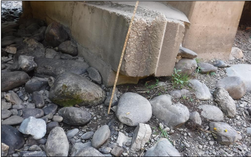
Pier 2 scour at upstream side.
