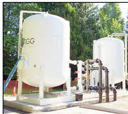
Figure 8. Pressure Filter Tanks for Adsorptive Inorganics Removal
