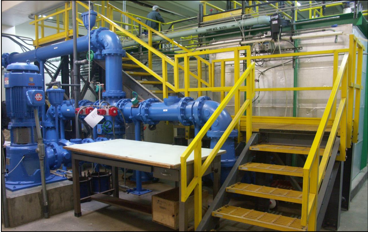
Figure 6. Example Packaged Treatment Units. Breckenridge, CO.
