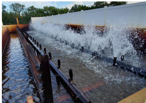
Figure 11. Example of Fountain Aeration of Iron
