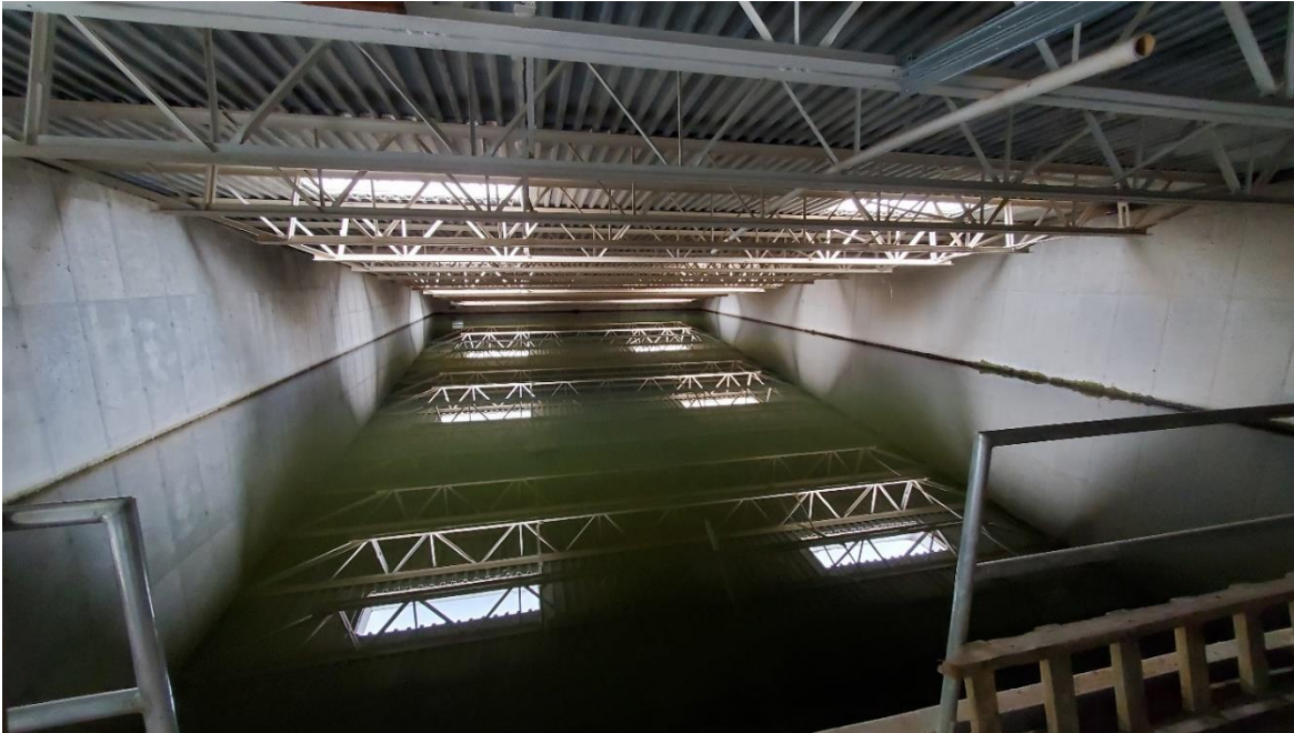
Figure 4. Minturn's Existing Slow Sand Filter (Filter 3)
