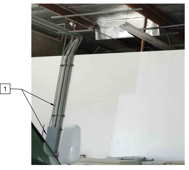
FRONT PICTURE OF EXISTING PANEL "P1" 2
