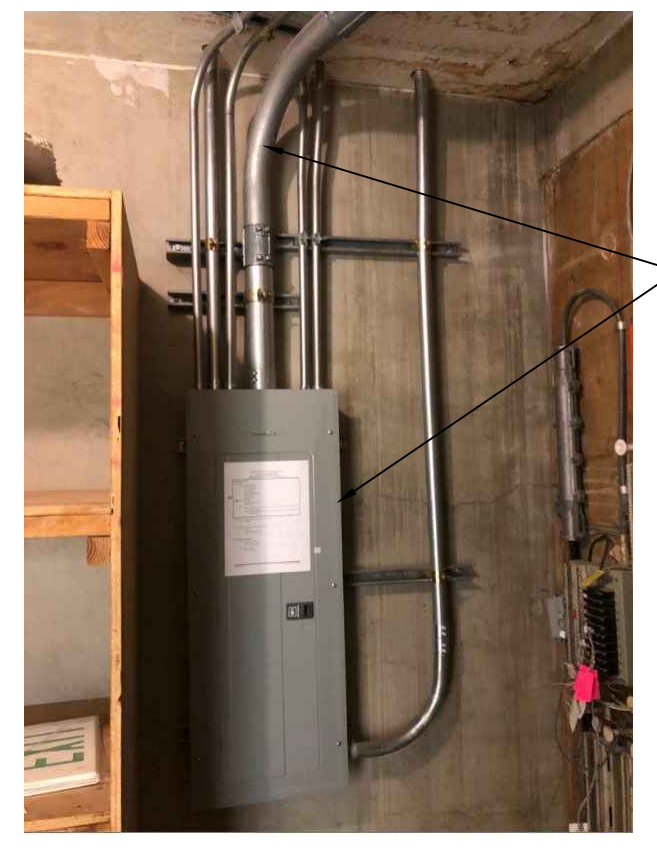
FRONT PICTURE OF EXISTING PANEL P3 3
