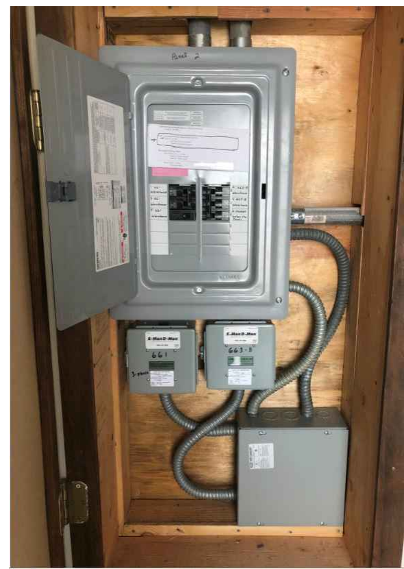
FRONT PICTURE OF EXISTING PANEL "P2" 5
