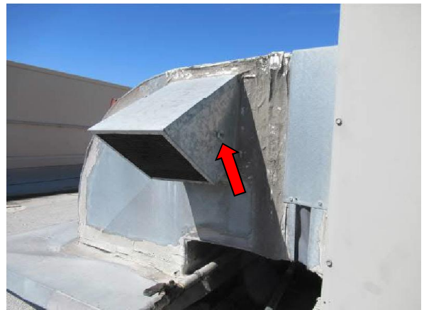
Photo #6 Typical adjustable outside air intake in the RTUs.
