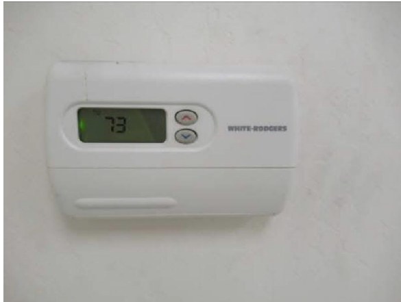
Photo #19 Typical wall mounted electronic thermostat.
