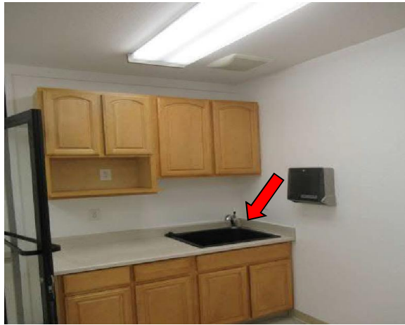
Photo #25 Example of code violation of industrial sink installed and provided with water pump to pump the drainage water out to the sink inside the janitor room.
