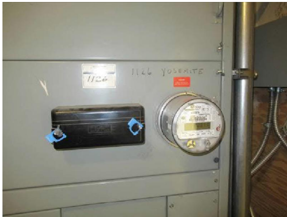
Photo #13 View of the main electrical meter.
