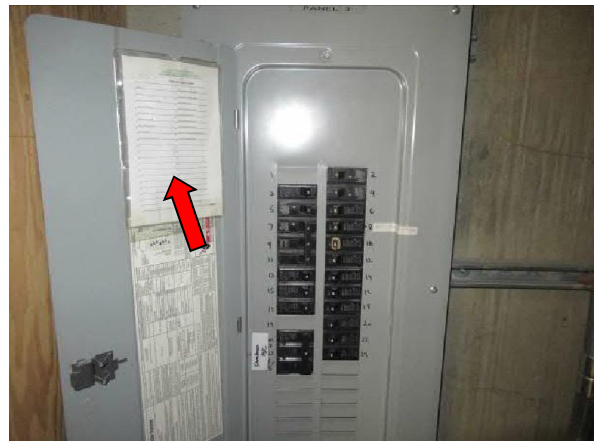
Photo #12 Typical electrical panel with index that needs to be updated.
