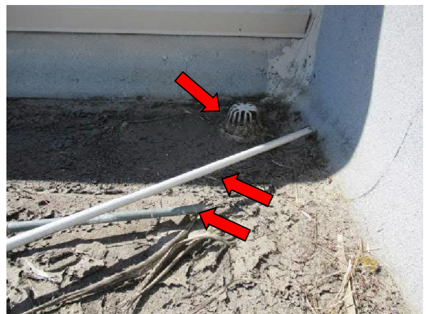
Photo #31 Example of a code violation of condensate drains free discharging the condensate water to the roof drains.
