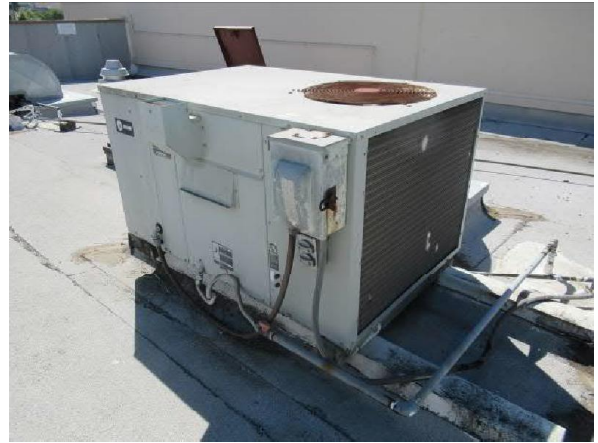
Photo #2 Side view of typical 3-ton RTU.
