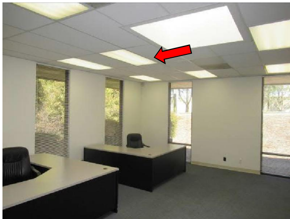
Photo #15 Typical T-8 fluorescent lights in the office space.
