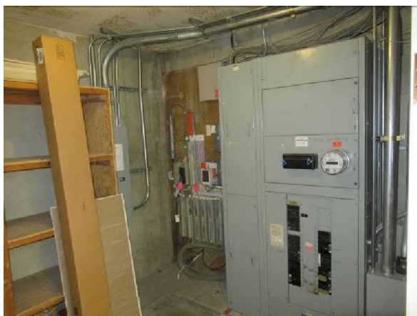
Photo #11 View of the main electrical main switch board in the electrical room.
