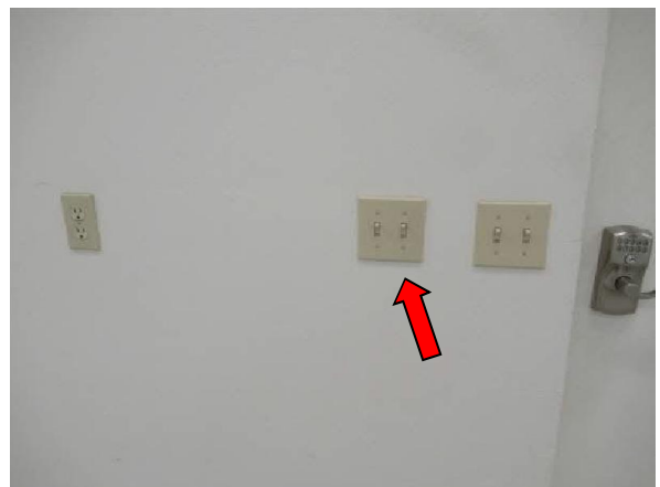
Photo #18 Typical lighting manual lighting switches.
