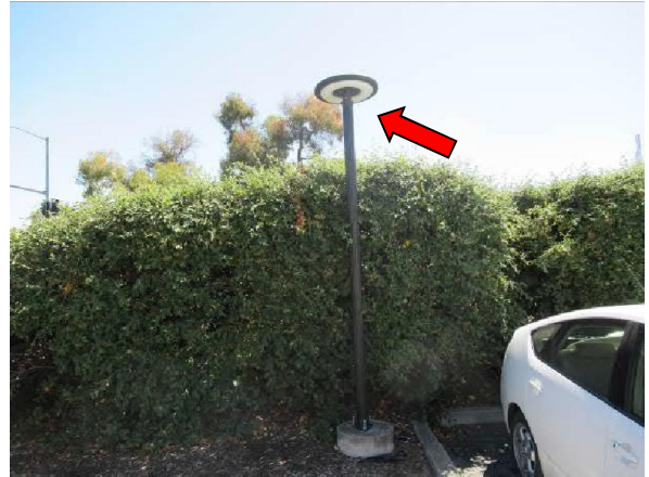
Photo #34 Typical external pole lighting fixture.
