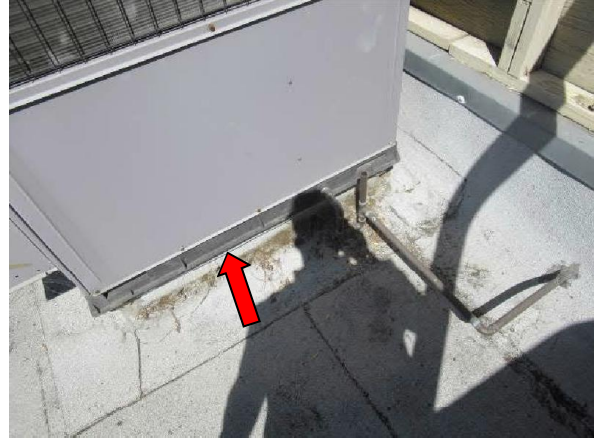
Photo #8 4-ton RTU is not provided with seismic restraint.
