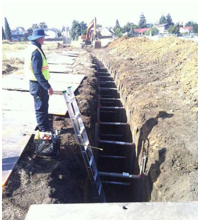
Photo 10: View of trench excavated by Geo-Logic Associates on behalf of Robson Homes for Alquist Priolo Special Studies Zone Investigation for the site. Photo taken in June 2015.
