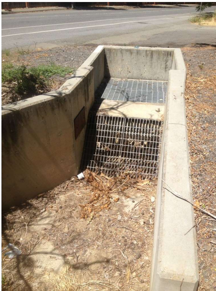
Figure 5-1: Trash and Debris Protection at Piedmont Creek Inlet
