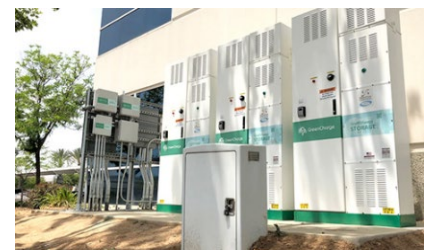
Figure 7. BESS at another ENGIE Project
