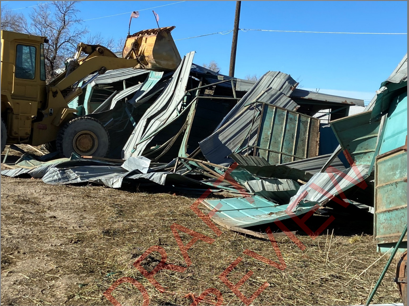
Photo: Straight Line Wind Damage, Natrona County Fairgrounds 2021
