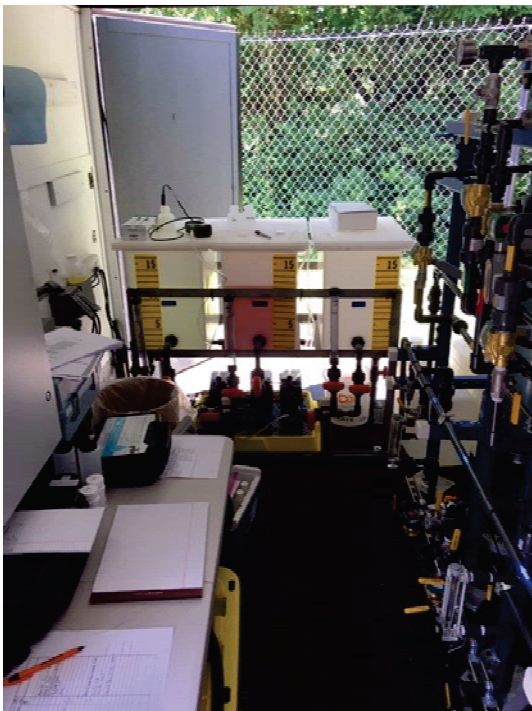
Photo 3. Reagent chemical pumping system
