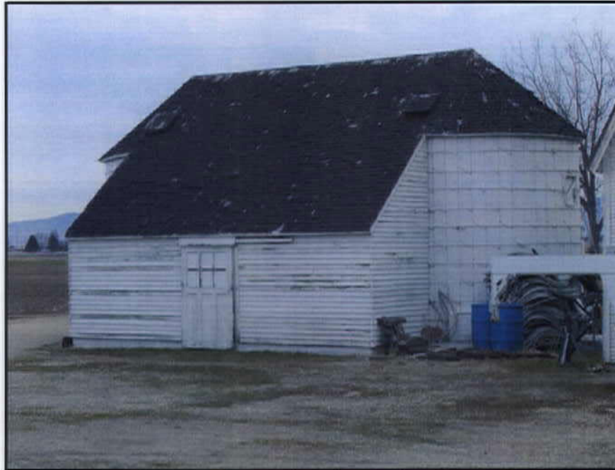
View looking northeast at the south and west elevations of No. 3 granary.
