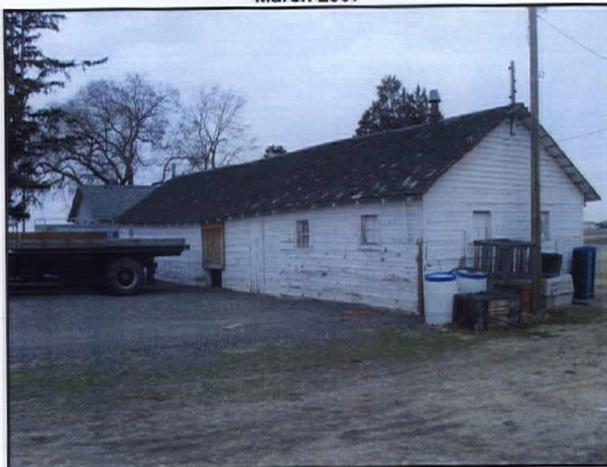
View looking northwest at the south and east elevation of No. 8 long shed.
