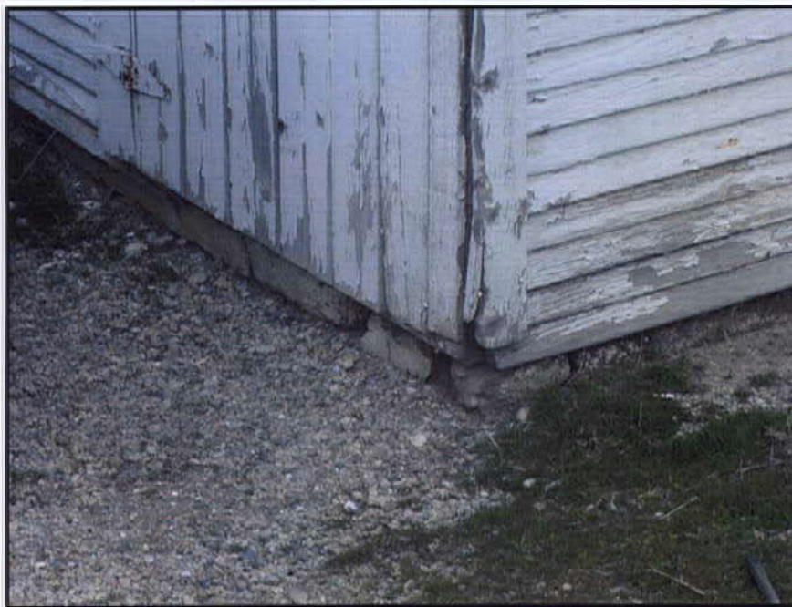
Close-up view of southwest corner of No. 4 barn, showing the use of quarried stone for the foundation.
