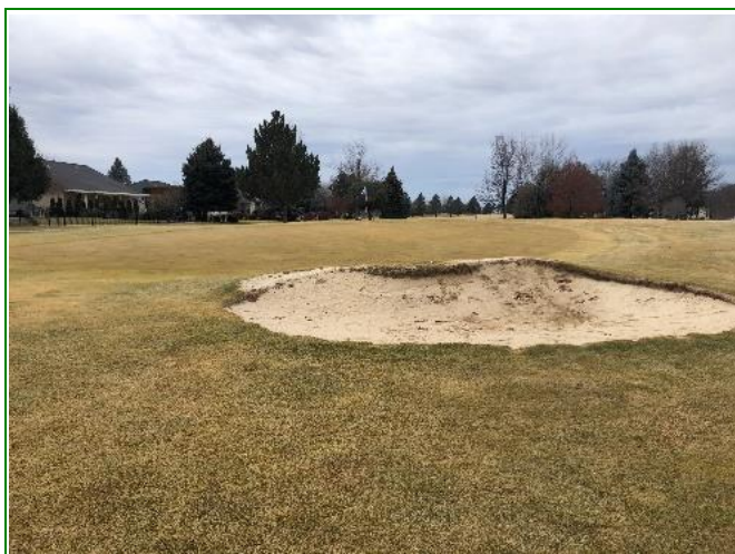
Sand bunkers are a hallmark of golf, adding both interest and challenge. All Lakeview GC sand bunkers are past their useful lifecycle and are in need of complete rebuilding, including sub-surface drainage, edging, and restored depth.
