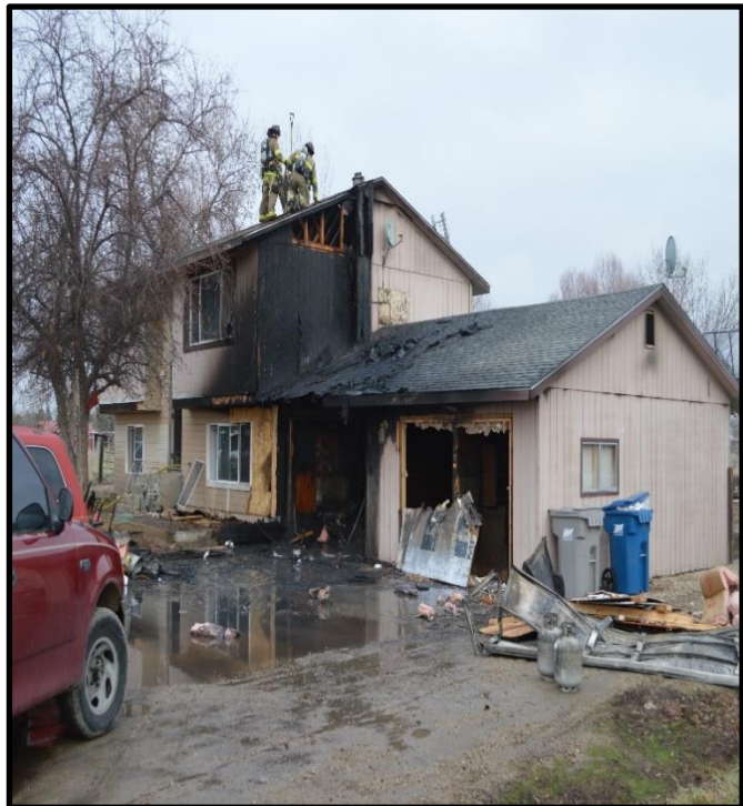
Fire Overhaul and Investigation
