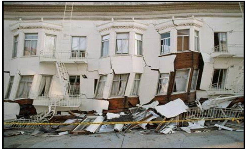
Earthquake Damaged Building (California)
