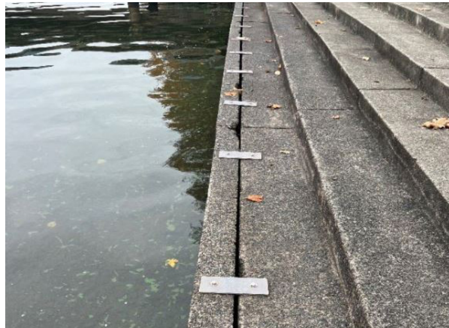
Facade separated from steps
