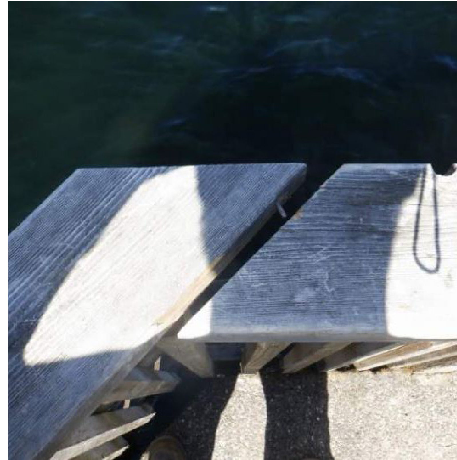
Failed railing connection
