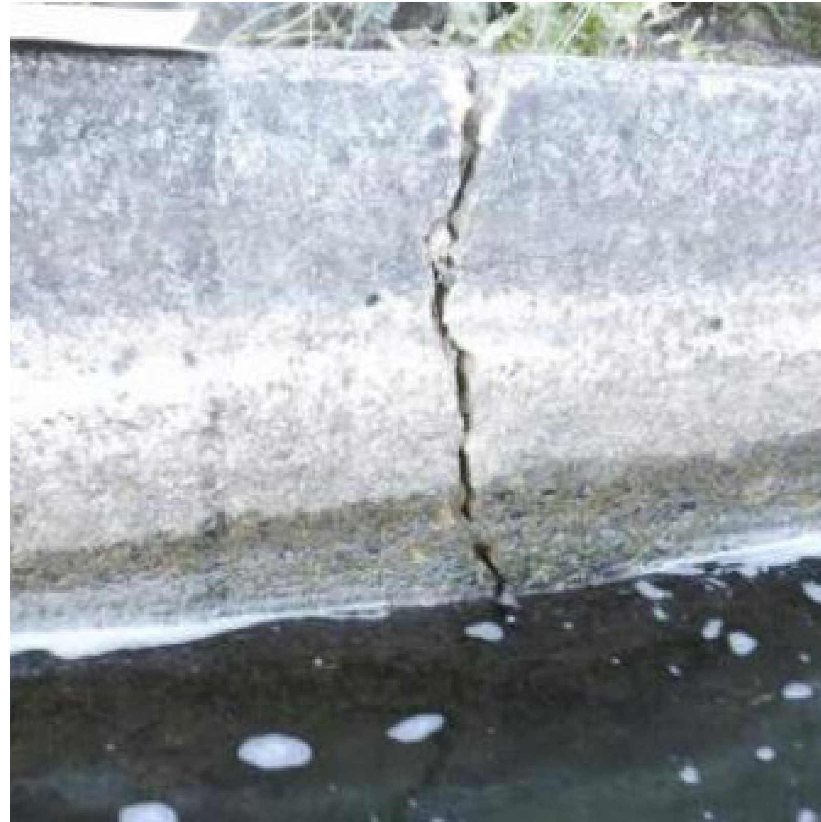
Cracked concrete bulkhead
