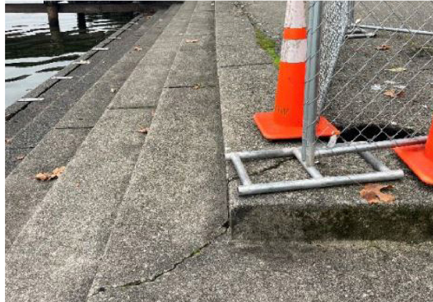
Cracked concrete stairs & sinkhole
