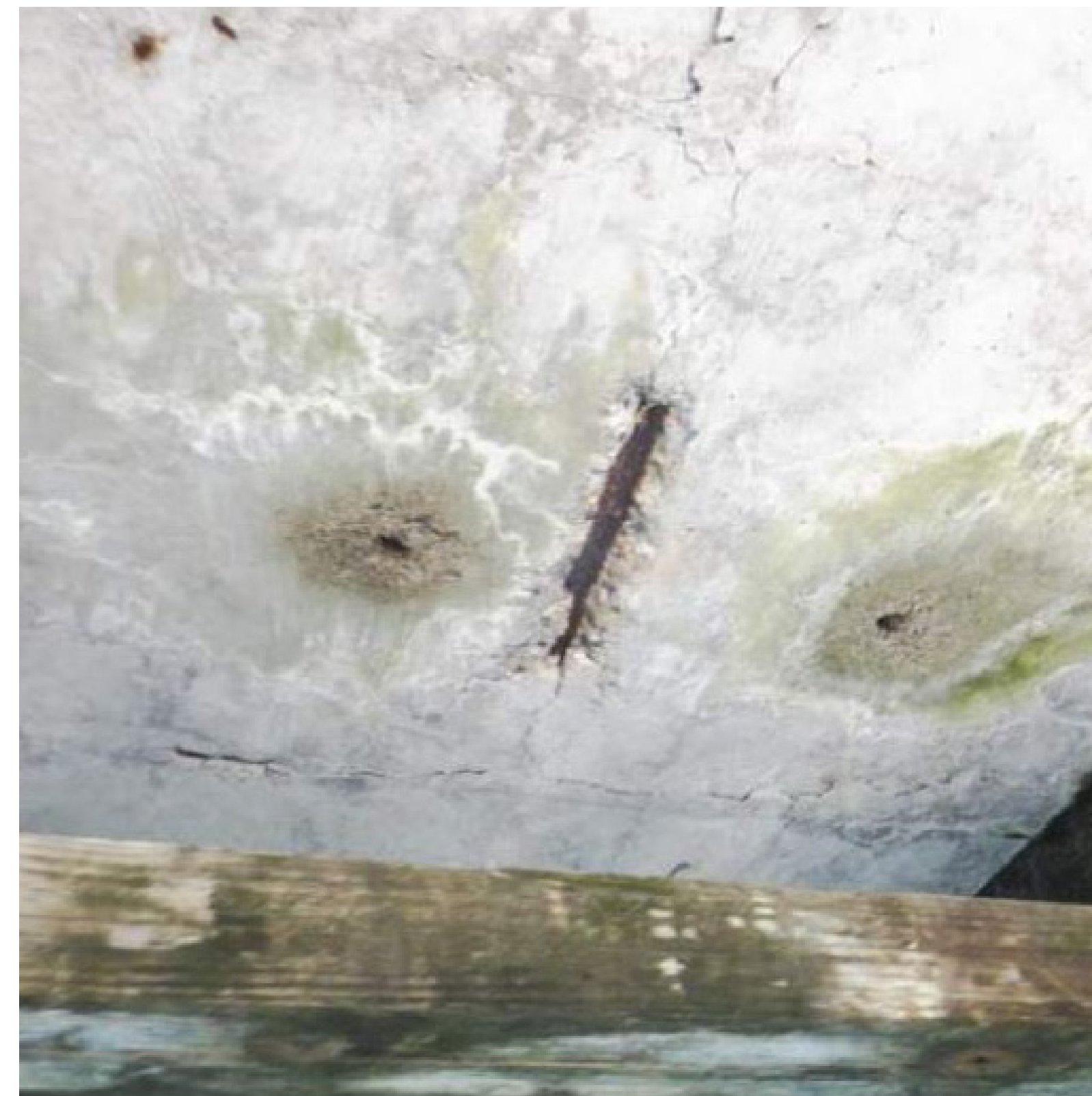
Delaminated, spalling reinforcement
