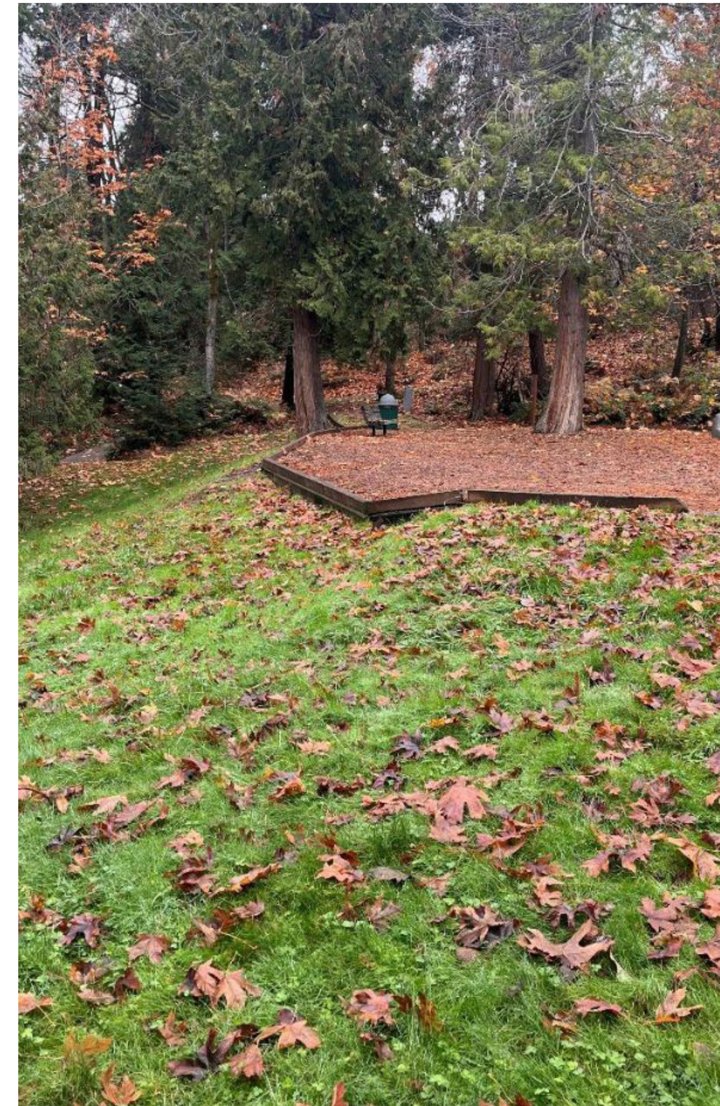
Soil creep causing mid-slope settling
