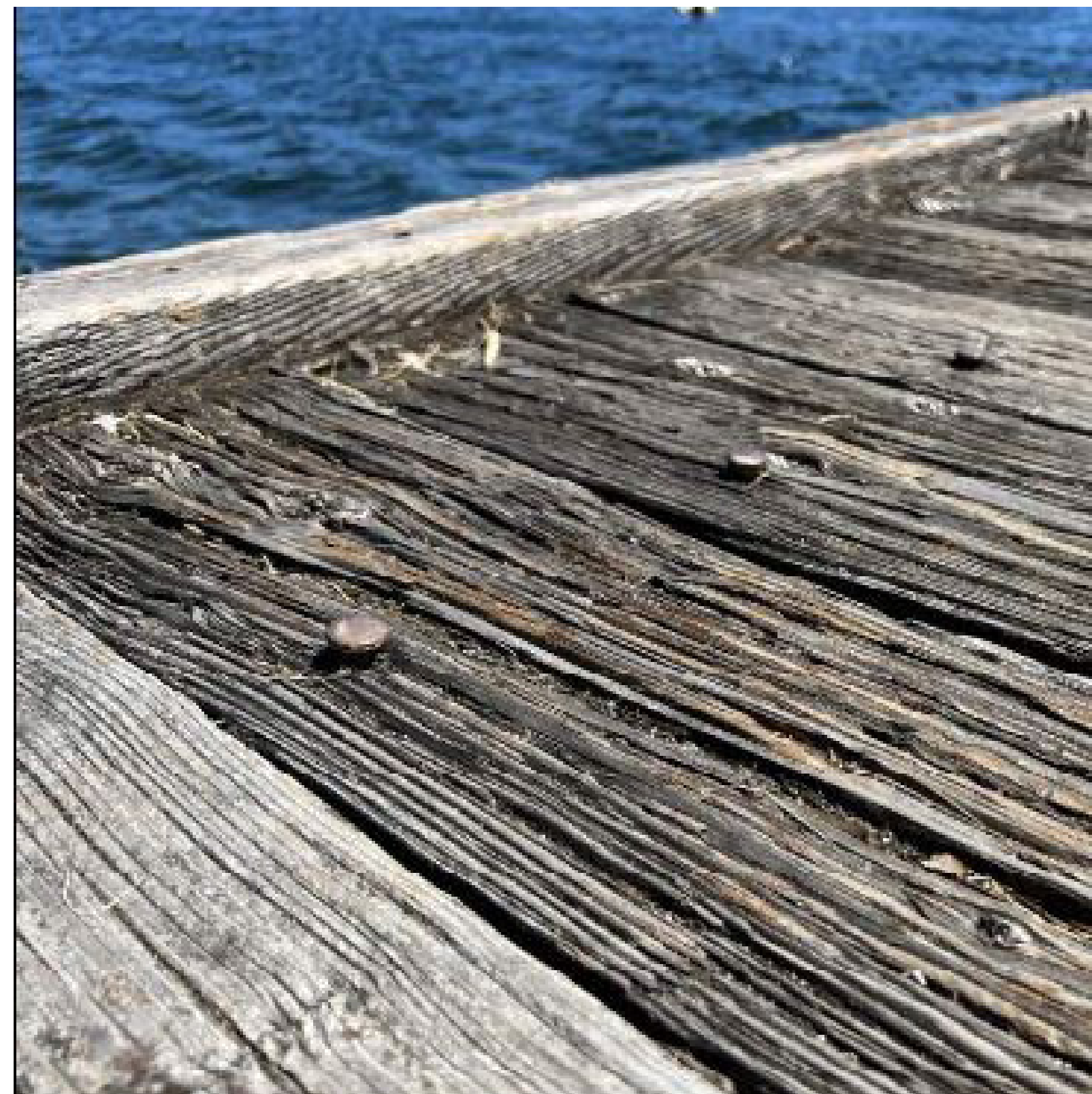
Typical worn, damaged decking
