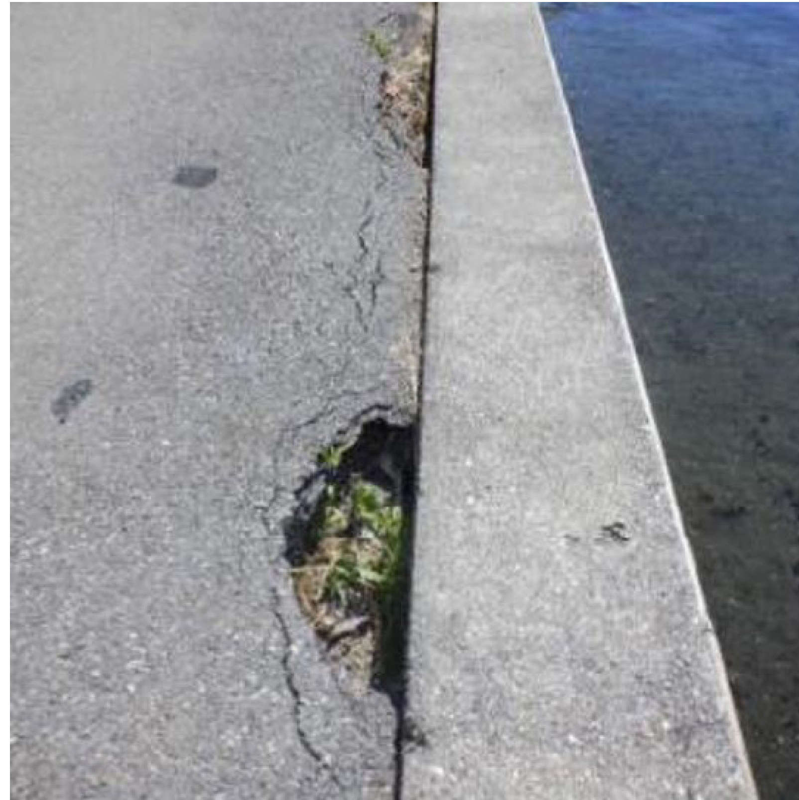
Sinkholes on swimming pier
