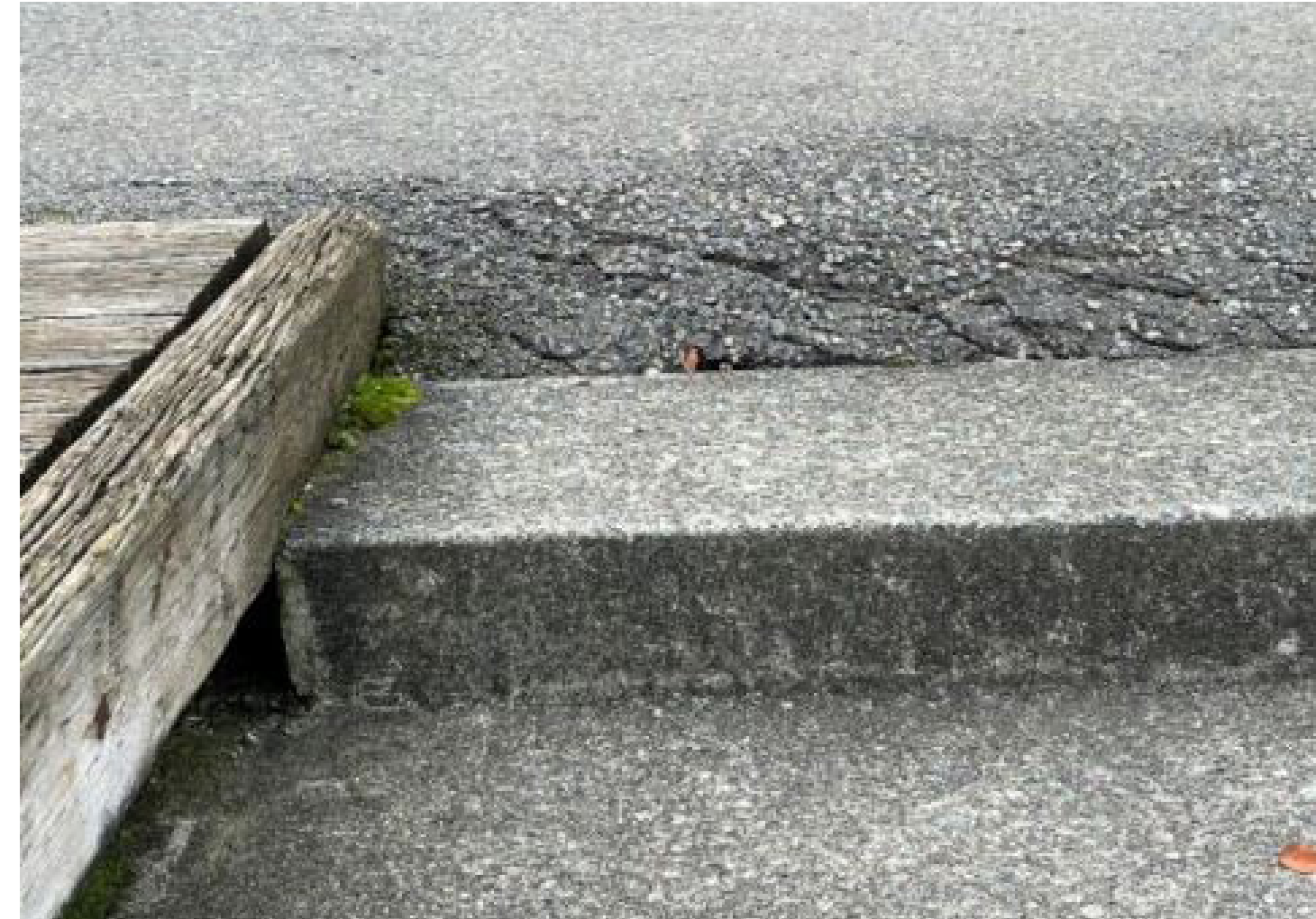
6" of settlement at south steps
