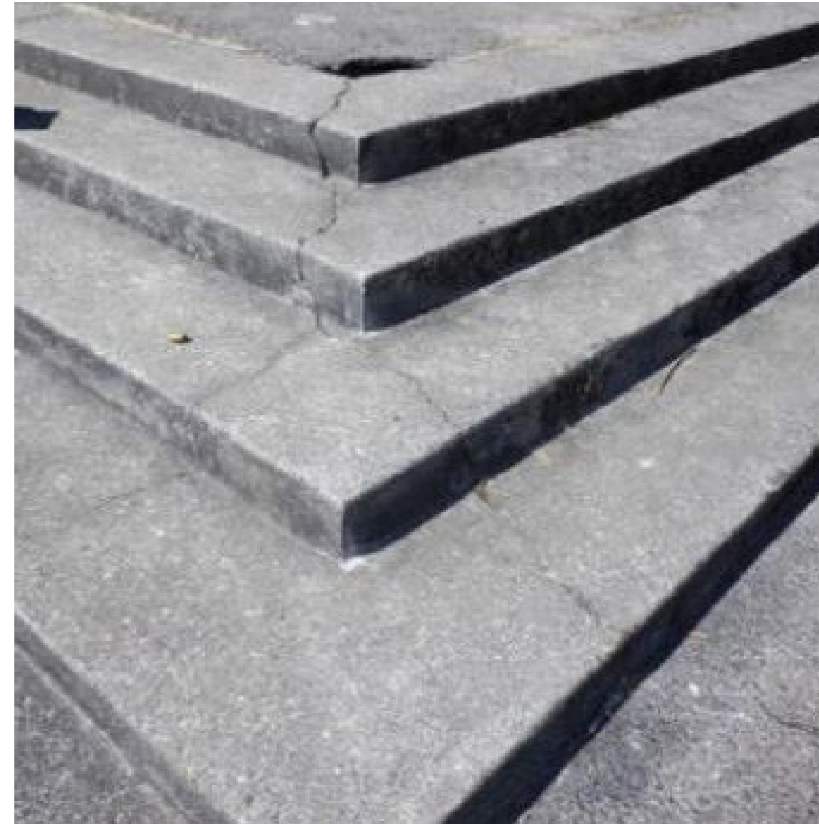
Cracked concrete stairs & sinkhole
