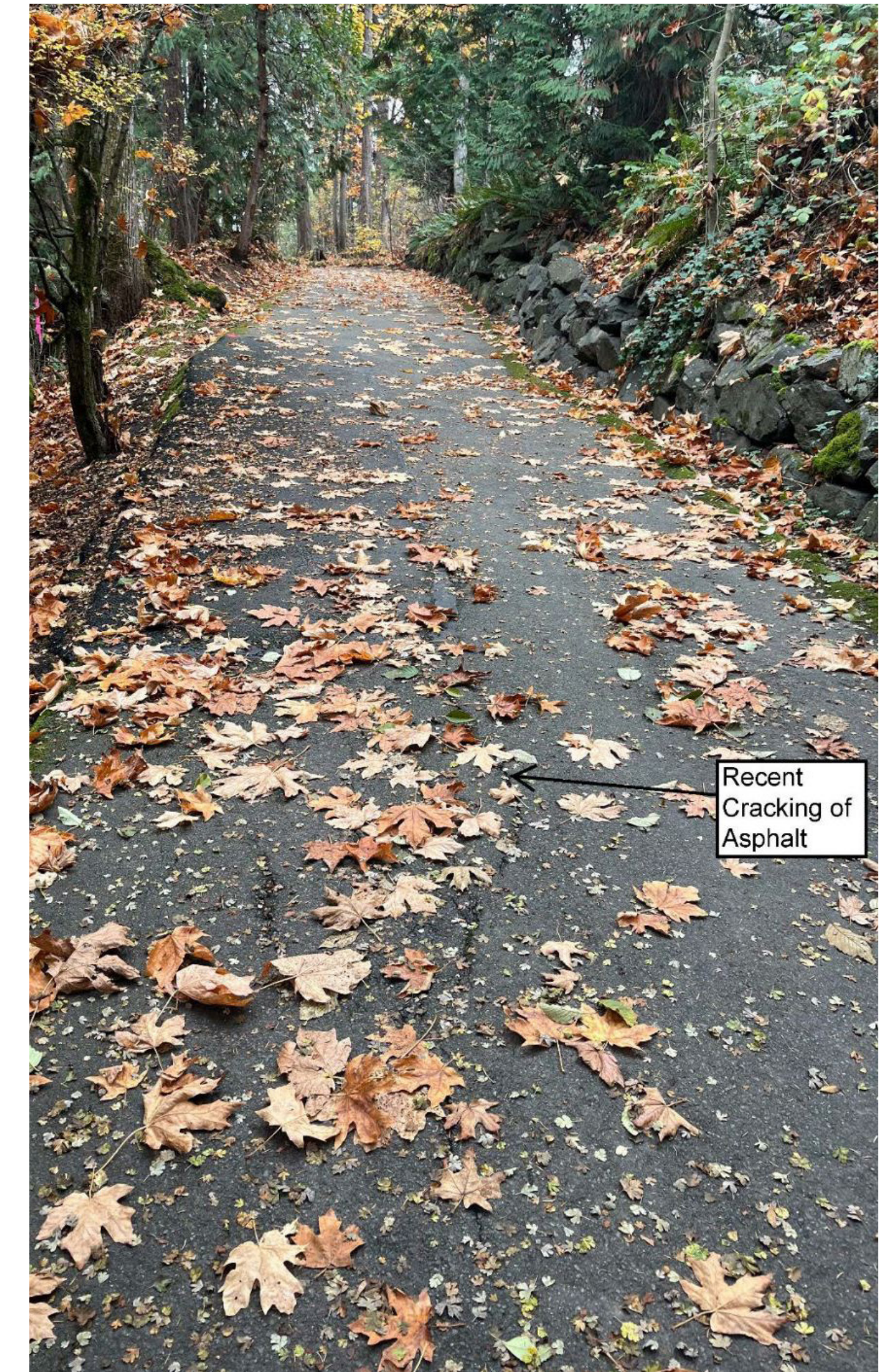
Recent cracking of asphalt
