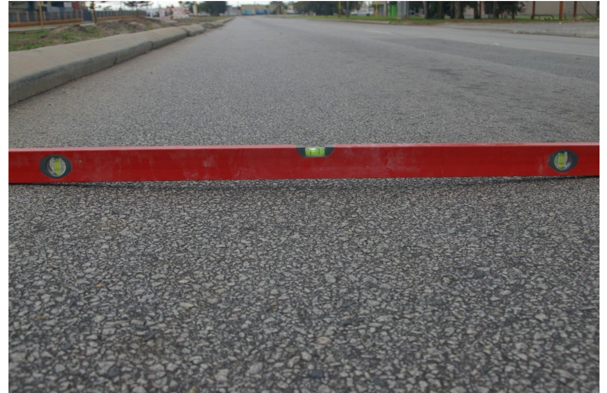
Rutting (wheel paths)
