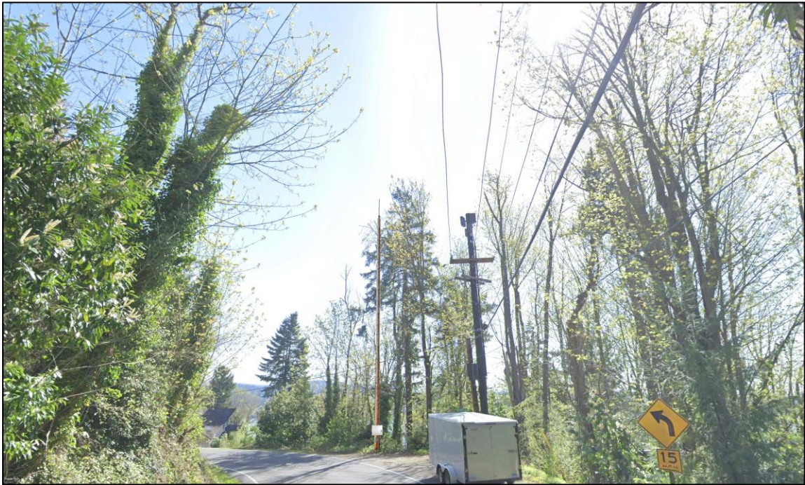
New 50' City-owned pole
