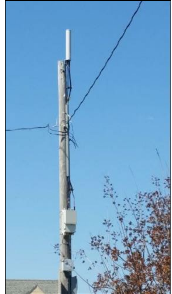
Example of antenna atop power pole
