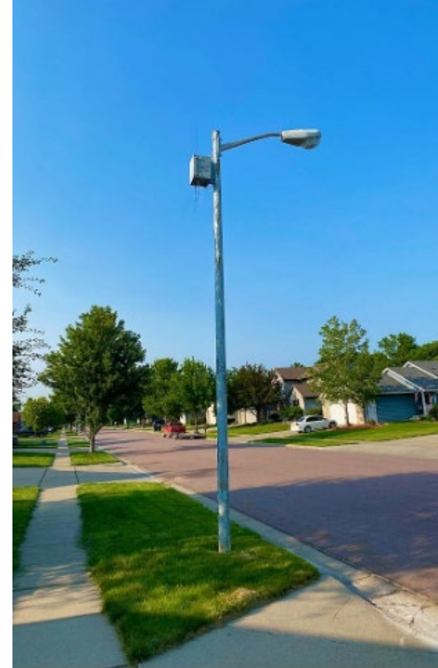
Example of small antenna on light post
