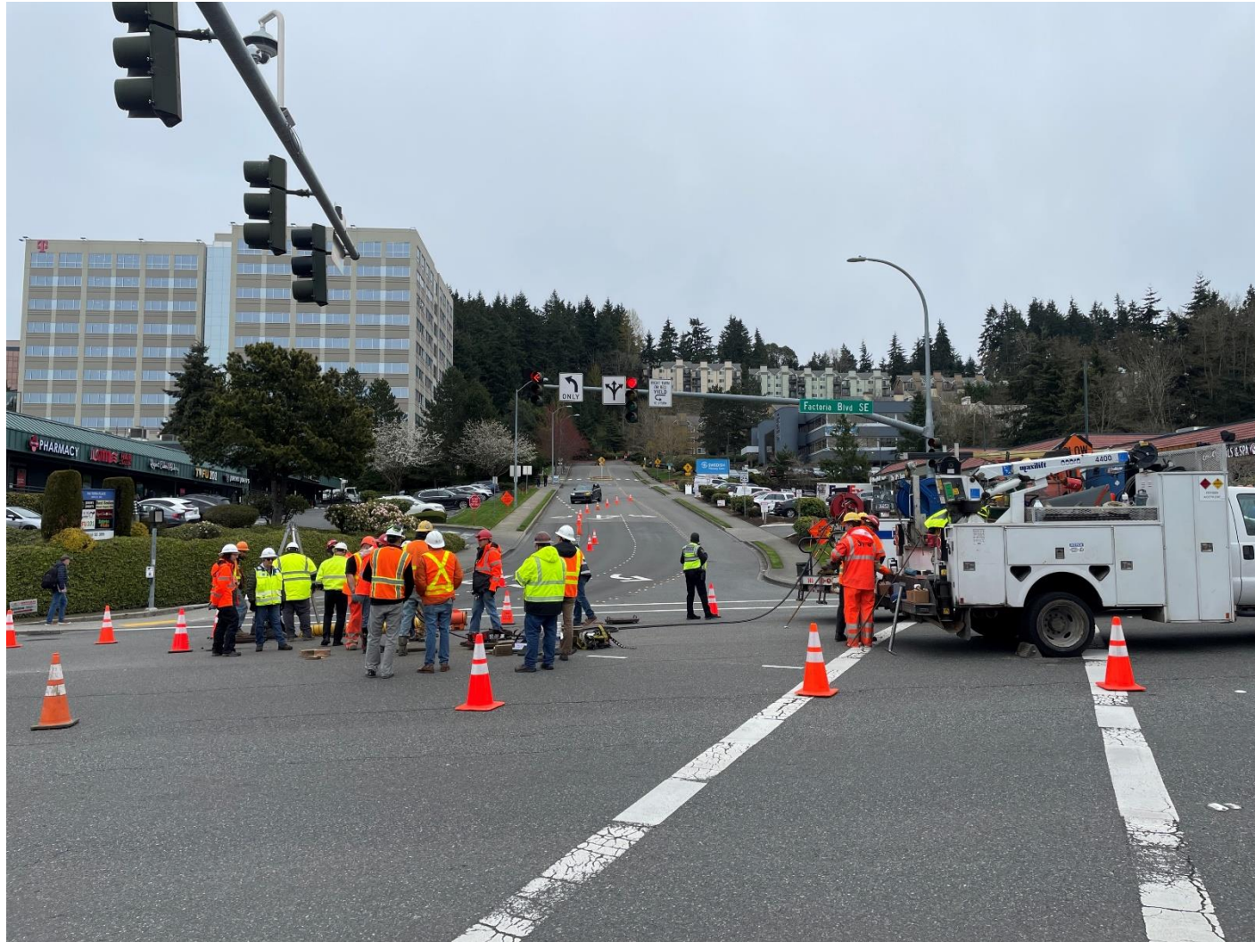
Valve that opened to 10% then froze is in the middle of the intersection in Factoria
