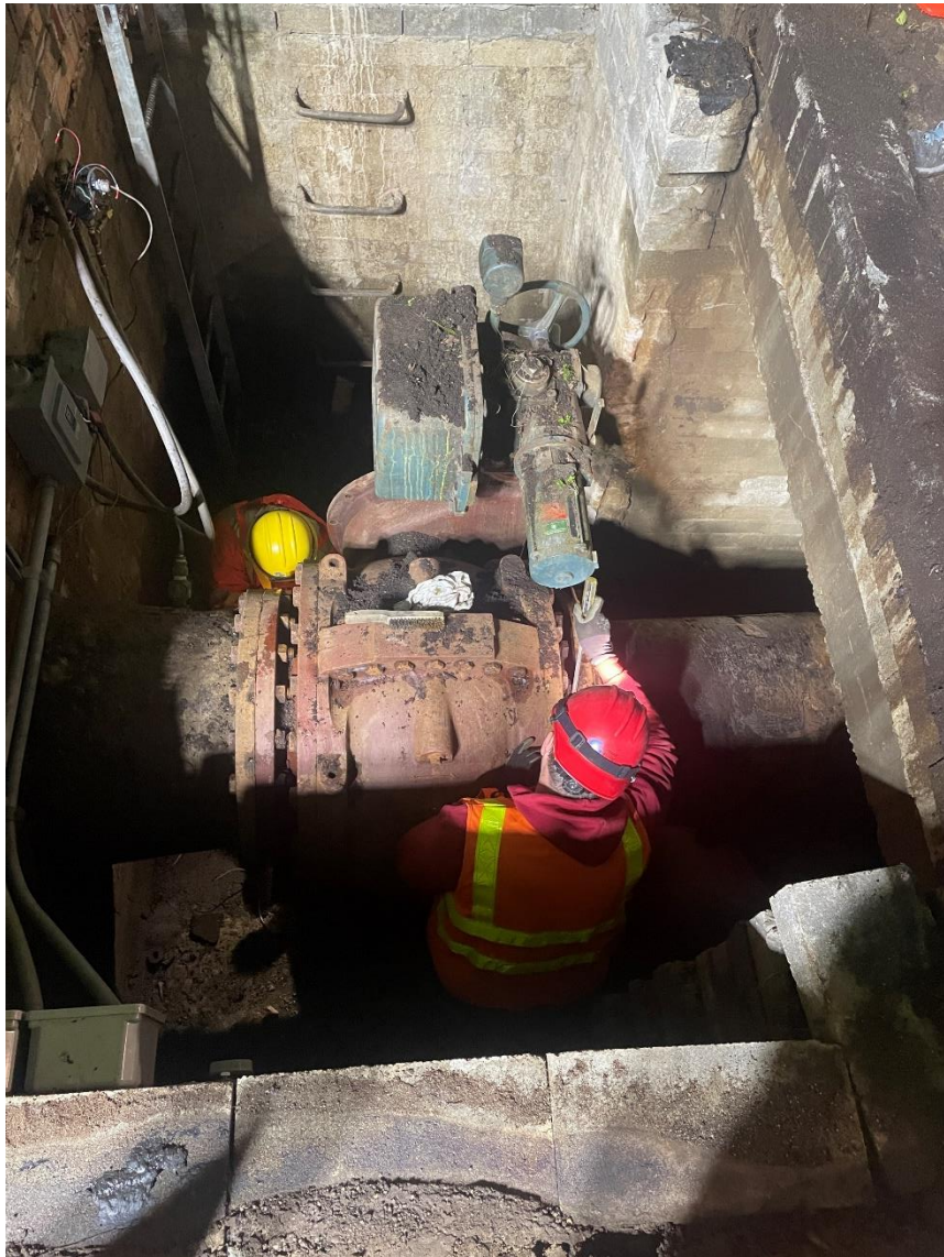
24-in ball valve that stuck closed
