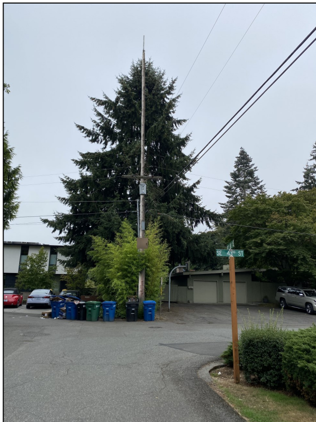
Photo rendering of example pole replacement in Crestwood area (94th Ave SE & SE 43rd St) with data collector equipment
