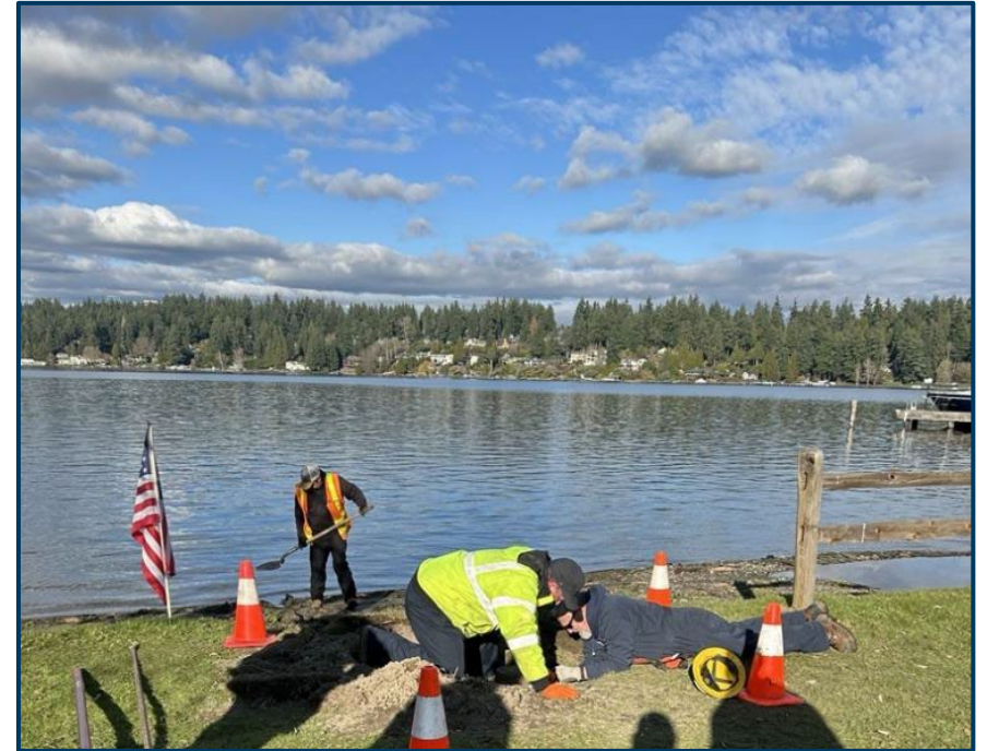
PW staff accessing the cap on the second access point to Pump Station 11.
