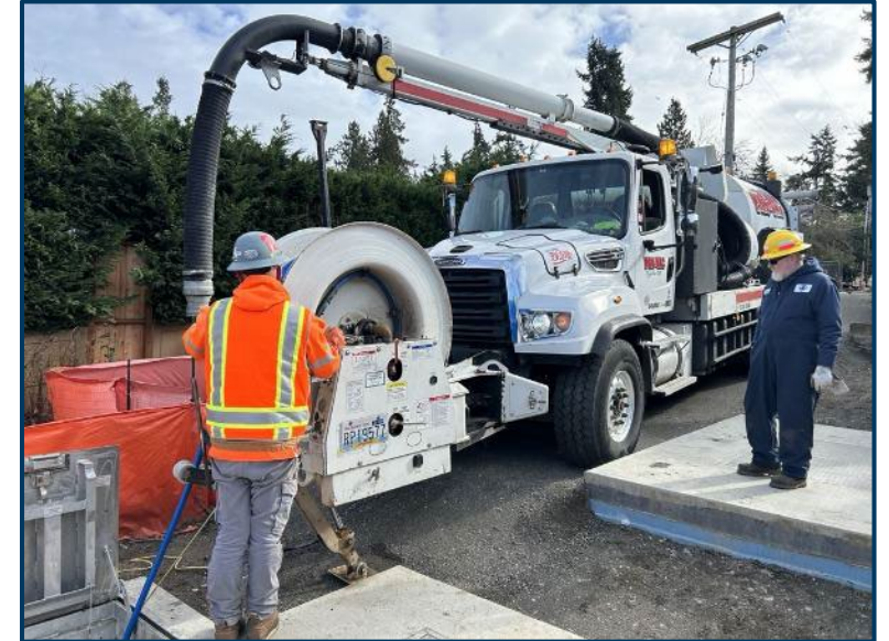
This is Pro Vac at Pump Station 11, jetting the lakeline west to the cleanouts at Covenant Shores.
