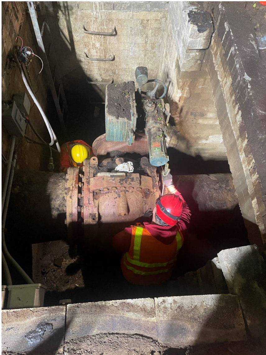
24-in ball valve that stuck closed
