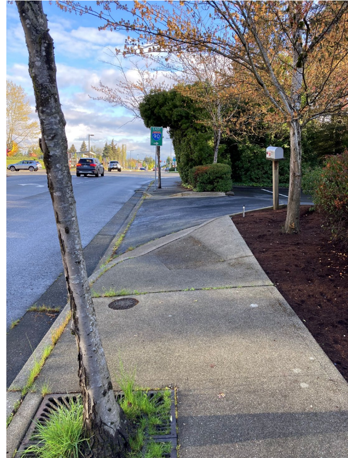
Poor ADA access at driveways
