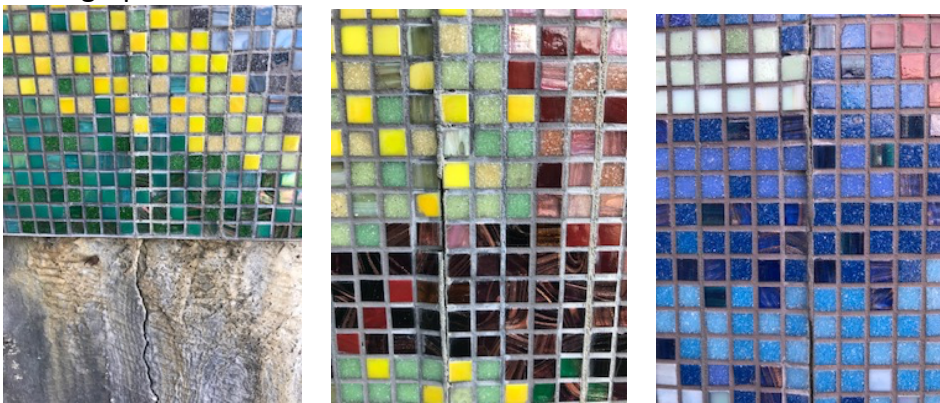
2019 – 2022: Notice how expansion joint shifts along the crack in the wall.
