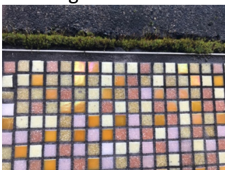
Moss and debris collect in the existing groove above the tiled mosaic.
