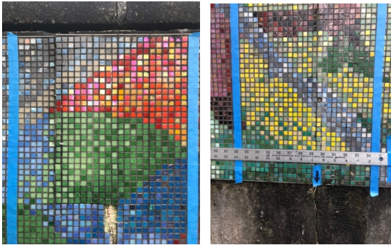
January 2024: The crack along the existing “fault line” has continued to expand causing more damage to the tilework.
