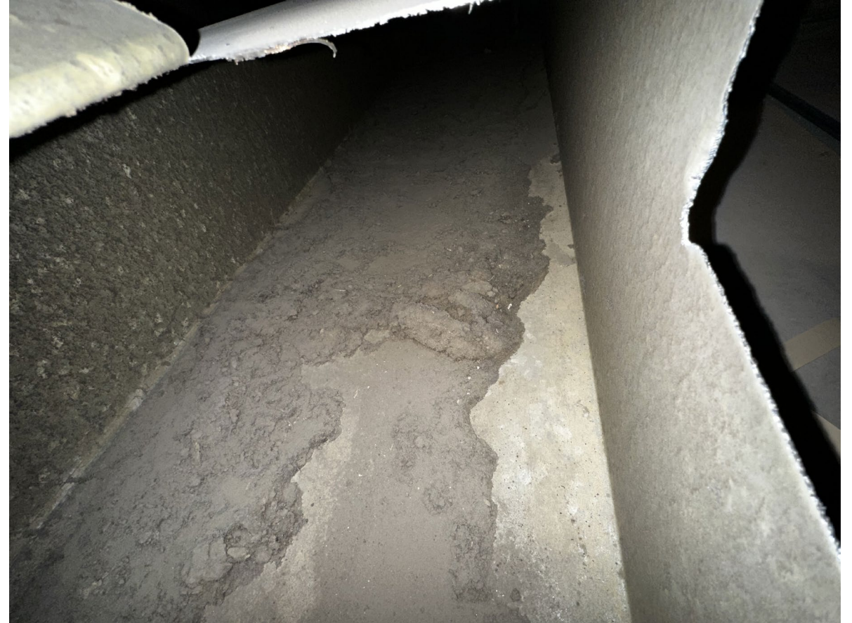
Picture: Dust build-up in an unlined duct in the attic mechanical room (sample D53).
