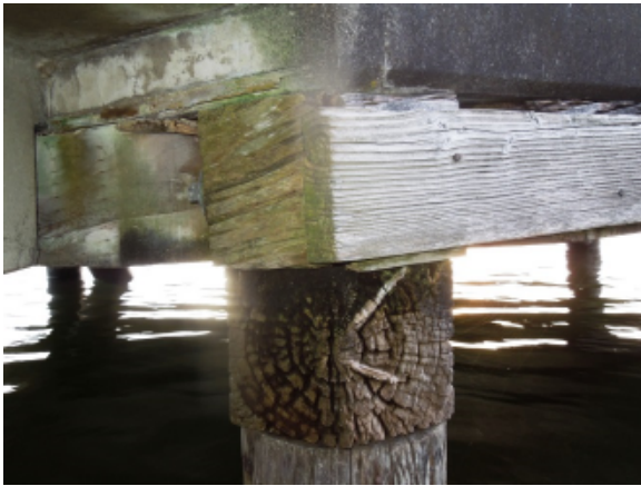
Photo 25A – Deteriorated cap beam (small pier)
