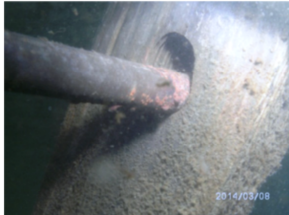
Photo 20A – Loose connector at substructure
