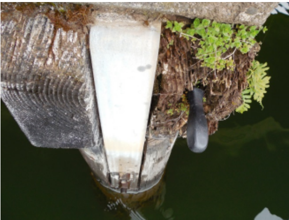
Photo 15A – Deteriorated cap beam end
