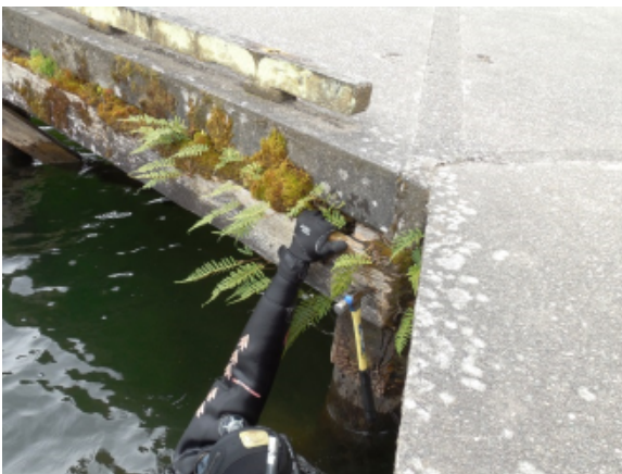
Photo 11A – Moss / vegetation at pier edge
