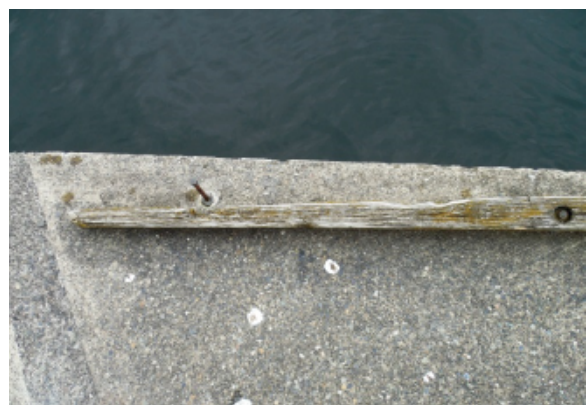
Photo 12A – Deteriorated / loose bull rail
