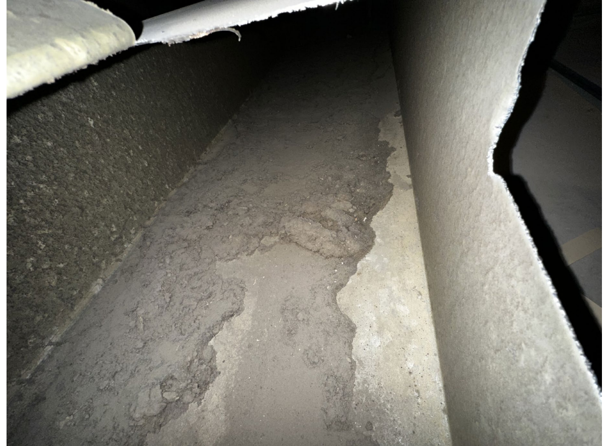
Picture: Dust build-up in an unlined duct in the attic mechanical room (sample D53).
