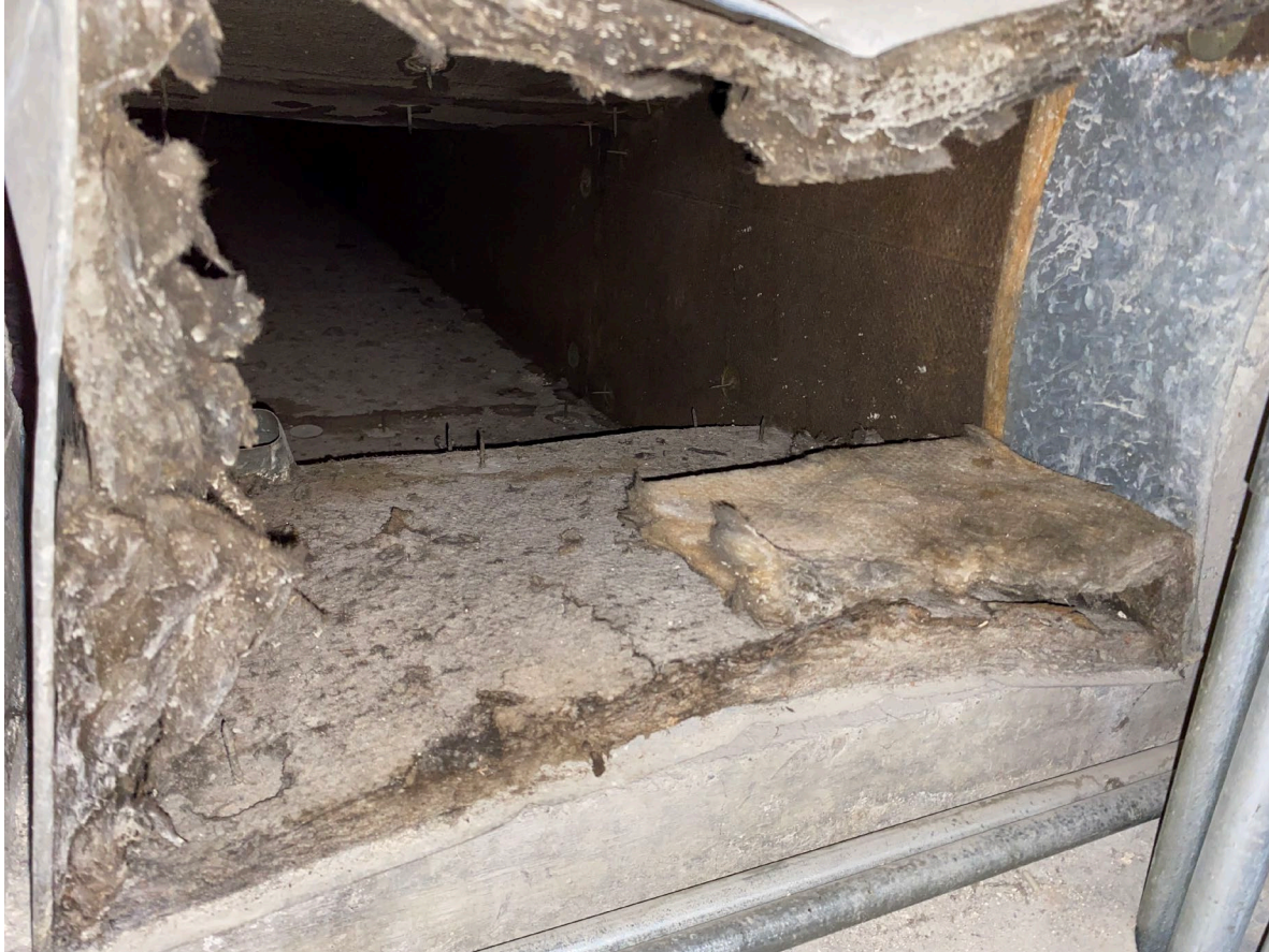
Picture: Example of lined duct in attic mechanical room.
